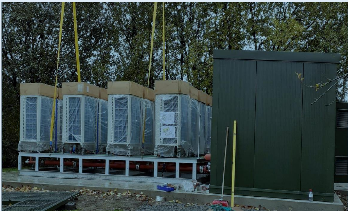
Communal Air Source Heat Pumps in Glasgow
