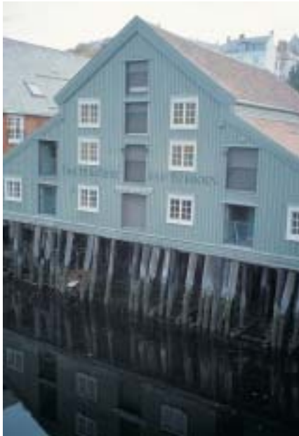
A converted warehouse in Trondheim, Norway is supported on wooden piles which are exposed to attack from marine borers and specialised fungi (Hazard Class 5). The timber cladding, although close, is at much less risk of biological degradation (Hazard Class 3).
