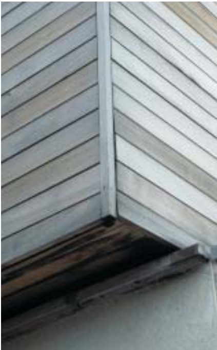
As the moisture content of the cladding has increased, the lack of expansion gaps in this western red cedar cladding has resulted in the boards bulging off the wall.
