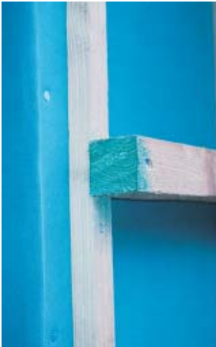
This batten has had to be cut to length on-site which has exposed untreated timber. In order to preserve the 'envelope of protection', the joiner has followed best practice by liberally coating the endgrain with a recommended preservative.
