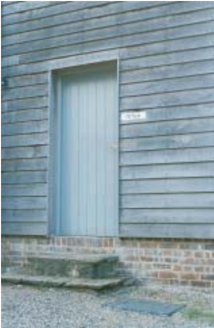
Elm cladding oversails the brick plinth to provide a gap for drainage and ventilation.
