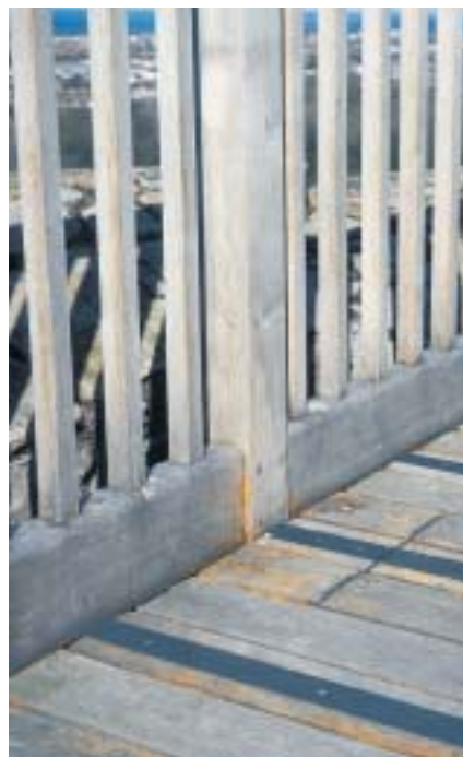
Oak external joinery with the remnants of a transparent coating which has failed after a couple of years. It would have been better not to have used a coating at all.
