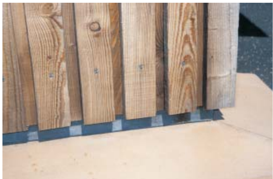
Timber should be kept above the 'splashline' - in this case the minimum 100mm has been used, although in most cases a larger gap of up to 250mm offers better protection.
