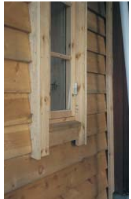
No attempt has been made to remove the (lighter coloured) sapwood of newly installed redwood cladding in Stavanger, western Norway. This cladding would subsequently have been painted with an opaque moisture vapour permeable coating.
