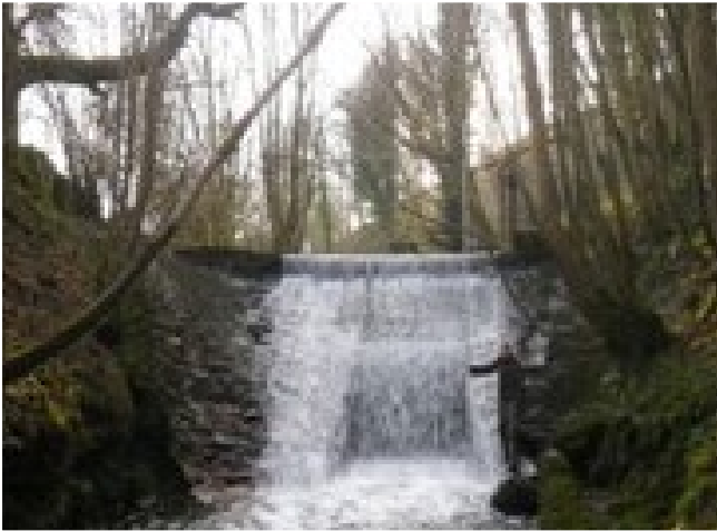
Tarff Creamery Weir before removal
