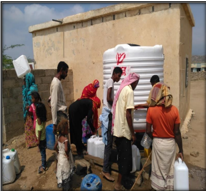
People from the IDP and Host communities queue for water at the water point constructed in Bura District.
