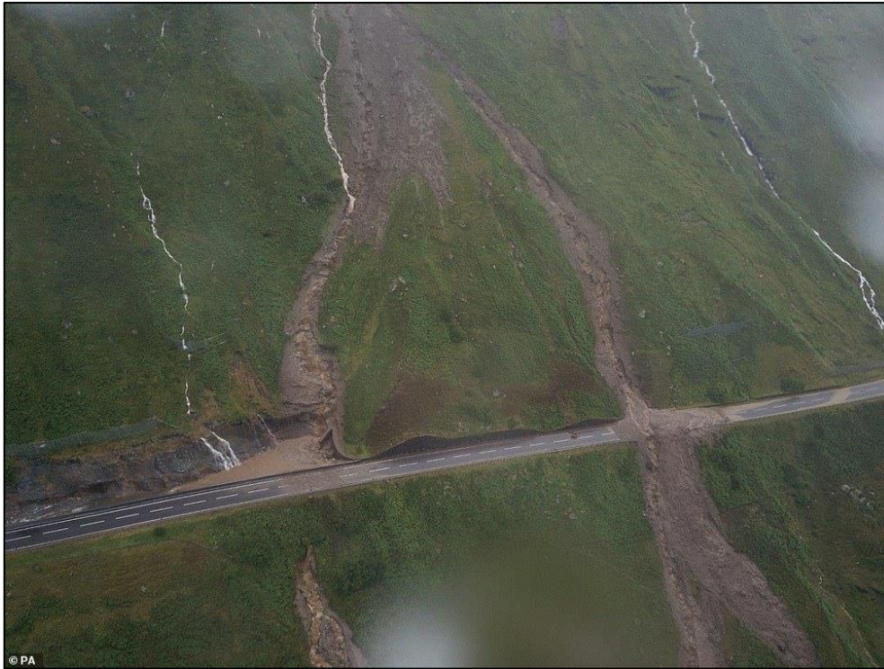
Figure 2: Photograph showing extent of August 2020 Landslip across A83
