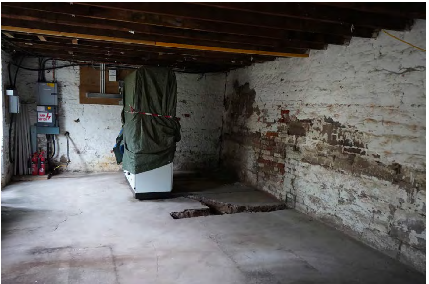
Bothy Building Interior - ground floor strip out and drainage channels cut in floor - MAY 2022
