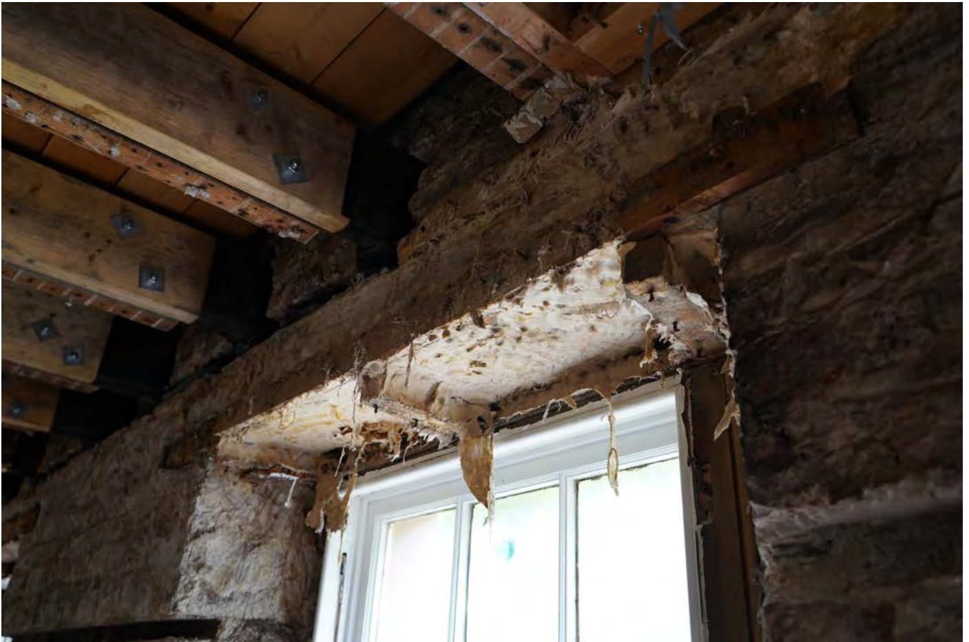
Bothy Building Interior - timber lintel removal due to dry rot and new concrete lintel to be installed - MAY 2022
