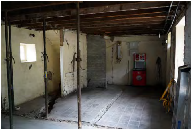
Bothy Building Interior - internal strip out and drainage channels cut in floor - MAY 2022
