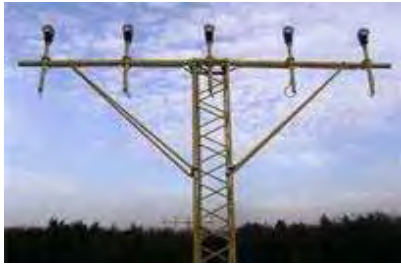
Electrically energised Navigation Lights for Sea and Air craft.
