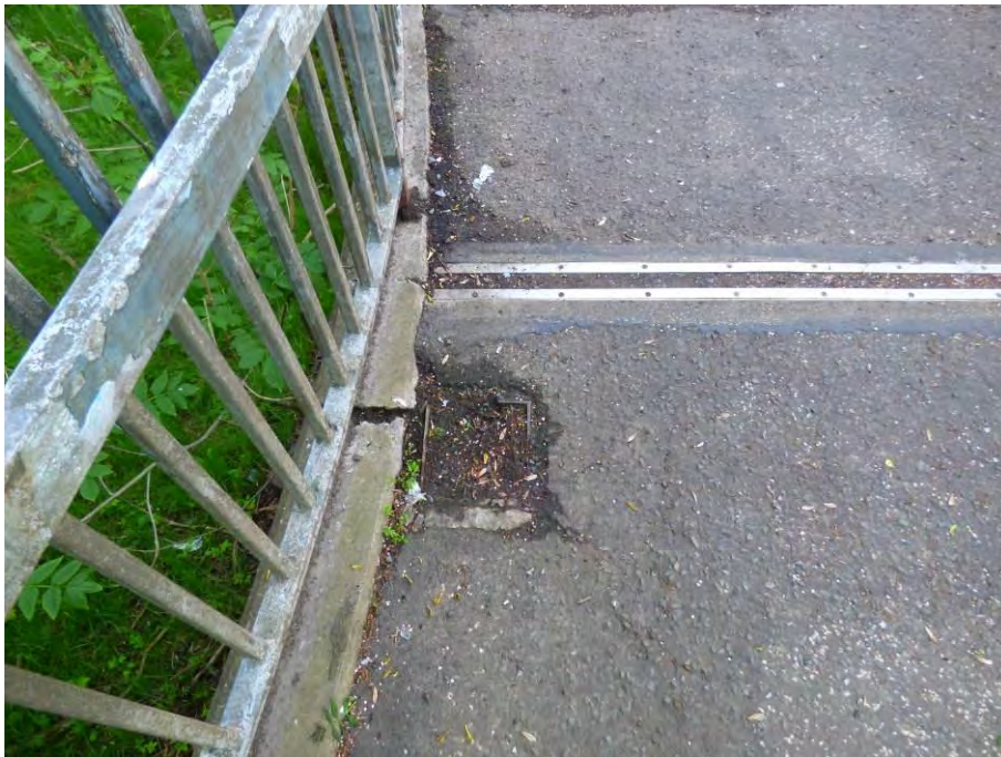
Photo 7 – LHS gully completely blocked at ES1 rail joint
