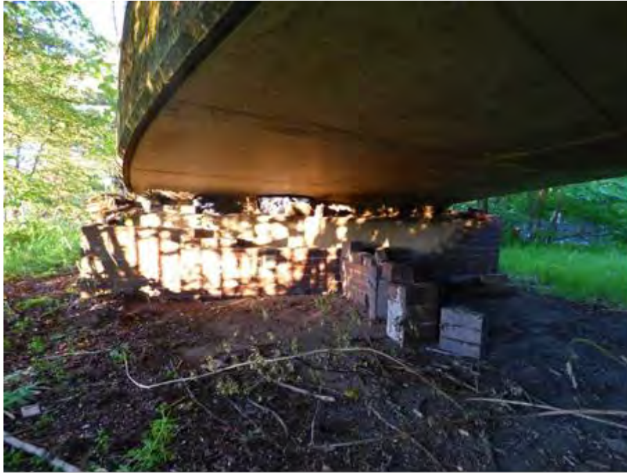
Photo 3 – Evidence of vagrant living on ES1 bearing shelf and brickwork façade damaged.
