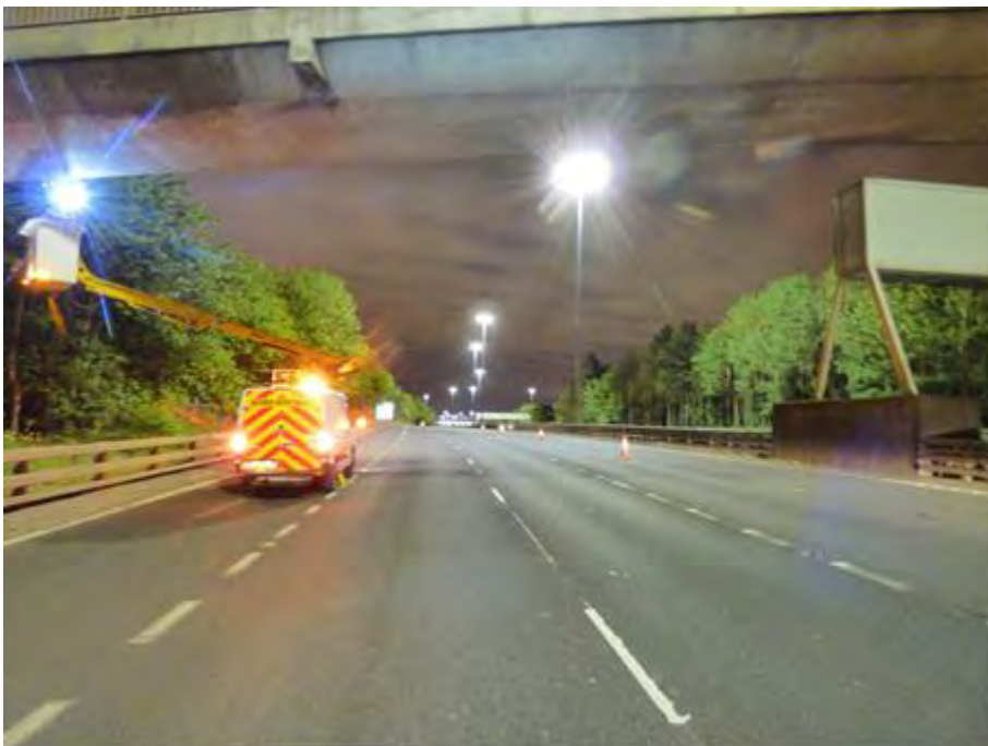
Photo 4 - VIEW LOOKING DOWNLINK M8
