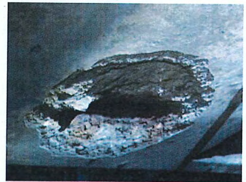
Second Main Defect
