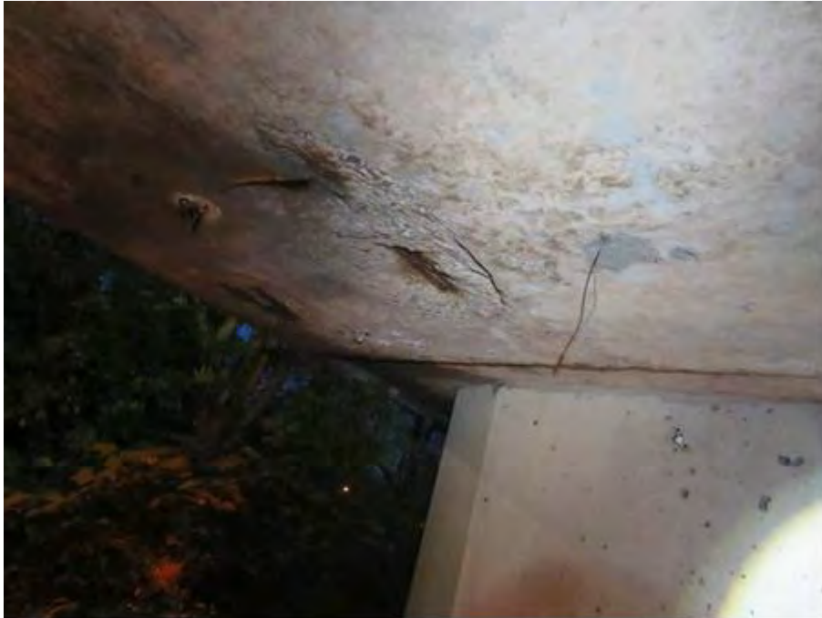
Photo 20 – Localised spall adjacent to IS8 half joint and span 7
