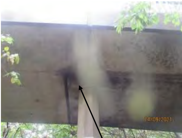
Photograph No. 1 - Minor localised spall on the IS8 half joint.
