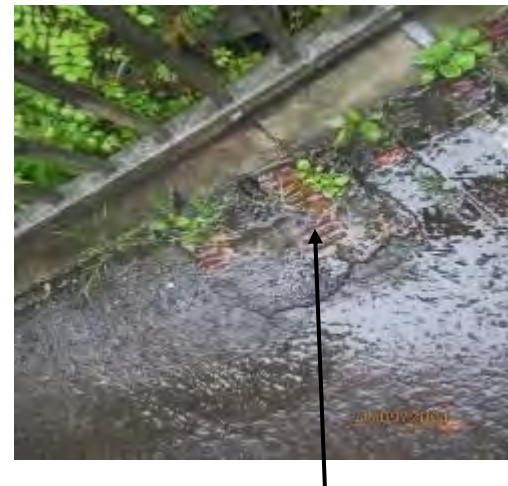
Photograph No.2 – Gully's totally blocked at ESP 13.
