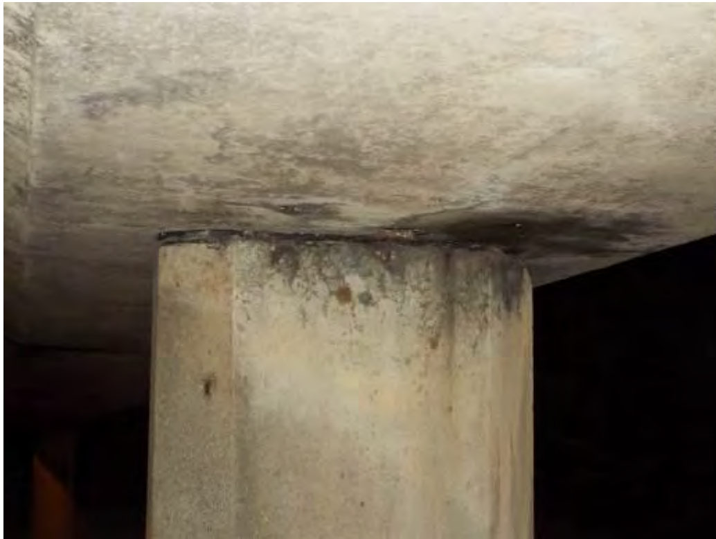
Photograph No.24 - Random cracking at top of ISP 3 on downlink face.
