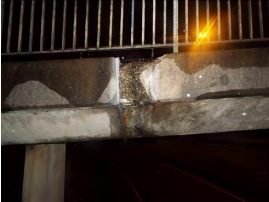
Photograph No.34 - Cracked / delaminated and spalled concrete on parapet upstand of half joint at uplink side of span No3 on LHS.
