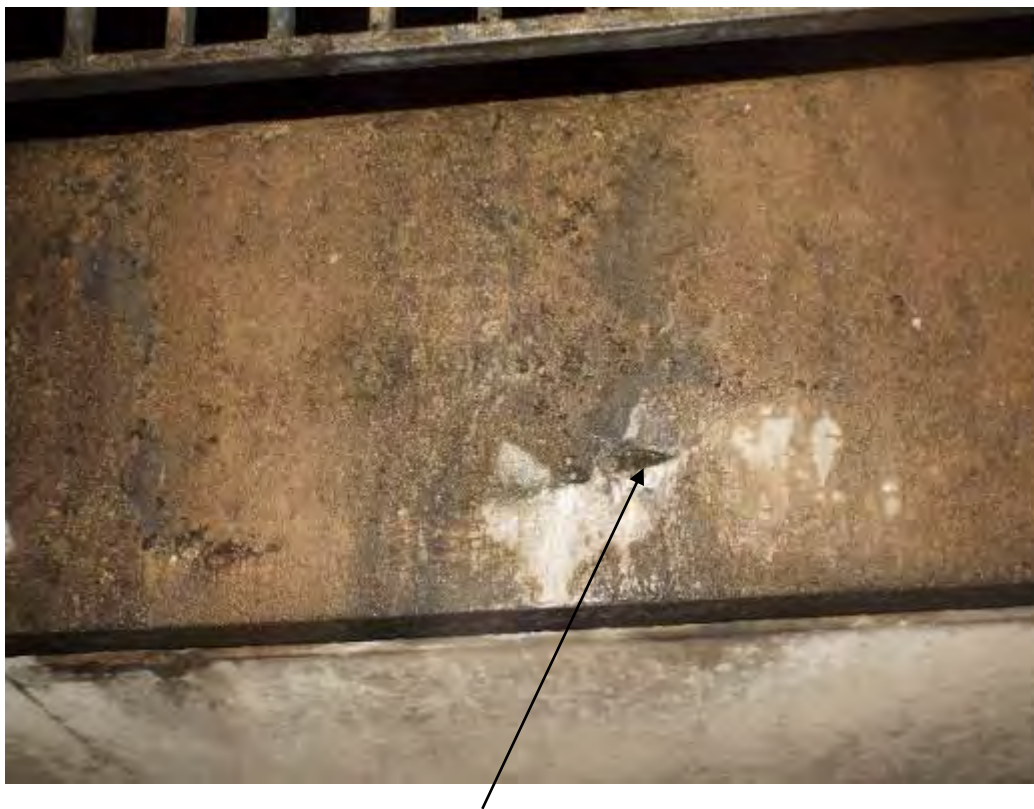
Photograph No.41 - Minor random cracking with 40mm void and leaching at LHS on parapet fascia.
