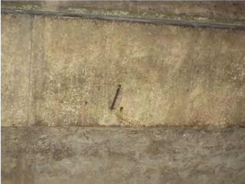
Photograph No.46 - Localised spall on deck slab exposing reinforcement at LHS of span No3.
