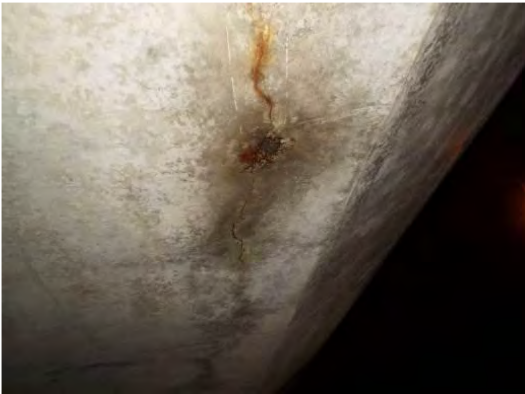
Photograph No.1 - (Typical) Longitudinal and horizontal cracking of reinforced concrete deck slab and soffit >0.3mm in places. Also rust staining which may suggest early signs of delamination.
