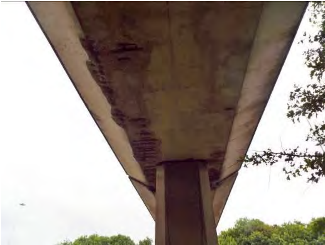
Photograph No.51 - Localised areas of spalled concrete on soffit and deck slab exposing reinforcement in span No4.
