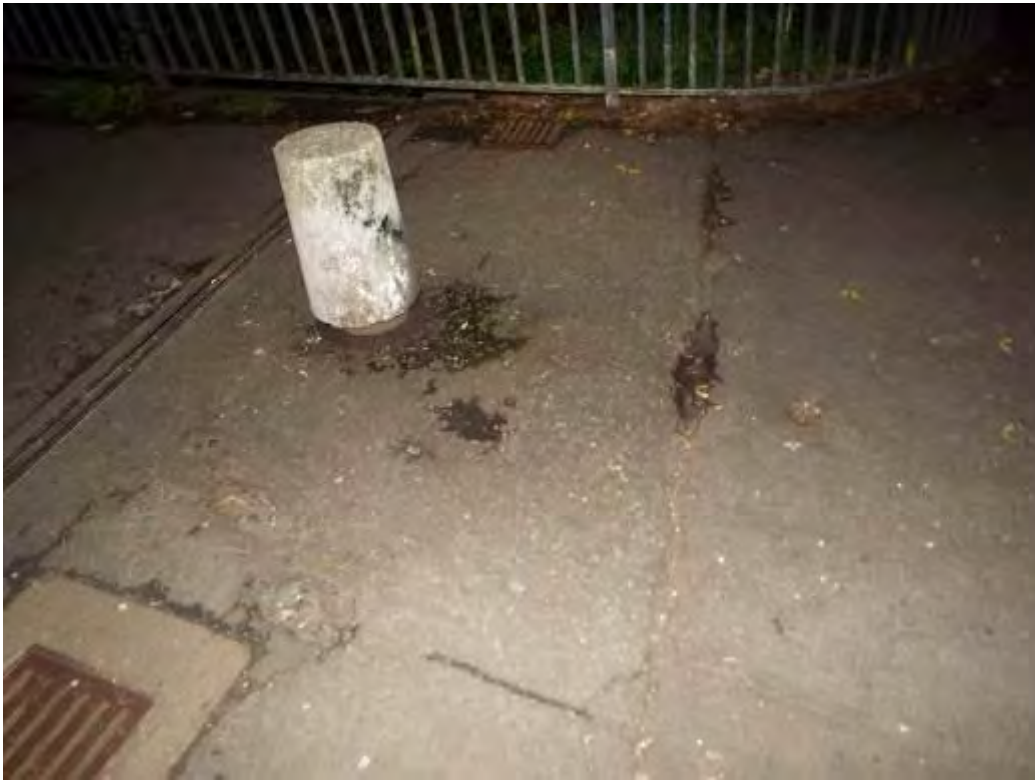
Photograph No.60 - Footpath surfacing appears to have been treated with road salts / grit making it uneven in areas.
