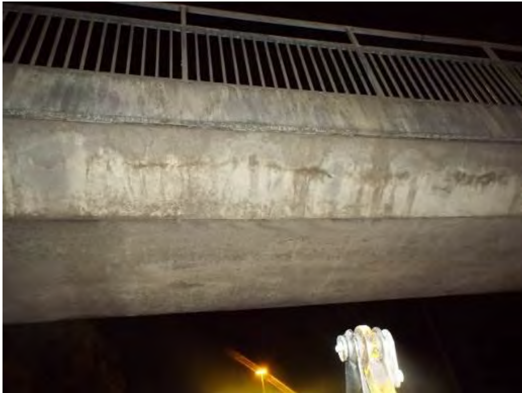
Photograph No.2 - (Typical) Longitudinal and horizontal cracking of reinforced concrete deck slab and soffit >0.3mm in places. Also rust staining which may suggest early signs of delamination.
