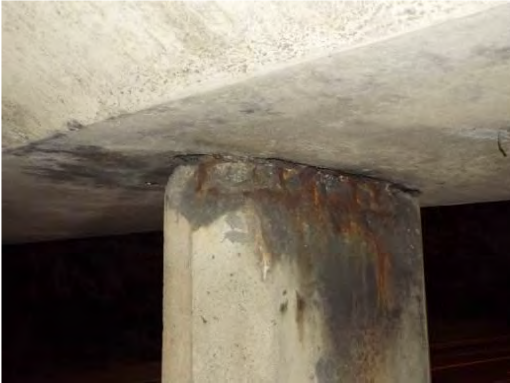
Photograph No.20 - Expansive corrosion of embedded reinforcement is resulting in rust staining at top of intermediate support No3 on uplink face.
