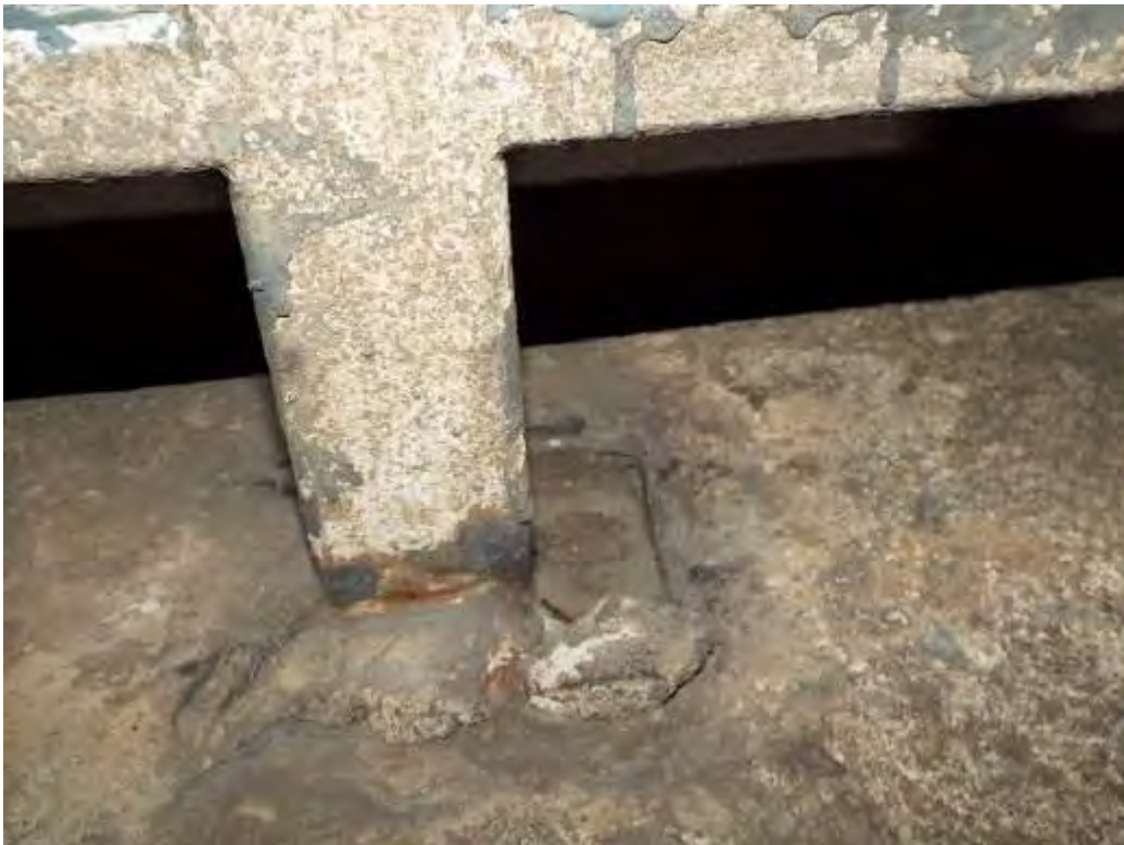
Photograph No.11 - (Typical) Localised areas of minor surface rusting on both parapet rails and post bases in all spans.
