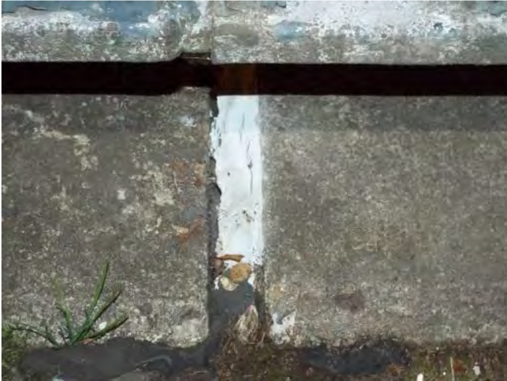
Photograph No.8 - (Typical) Polysulphide sealant de bonded at both sides of ESP 1 and half joint in span 1.
