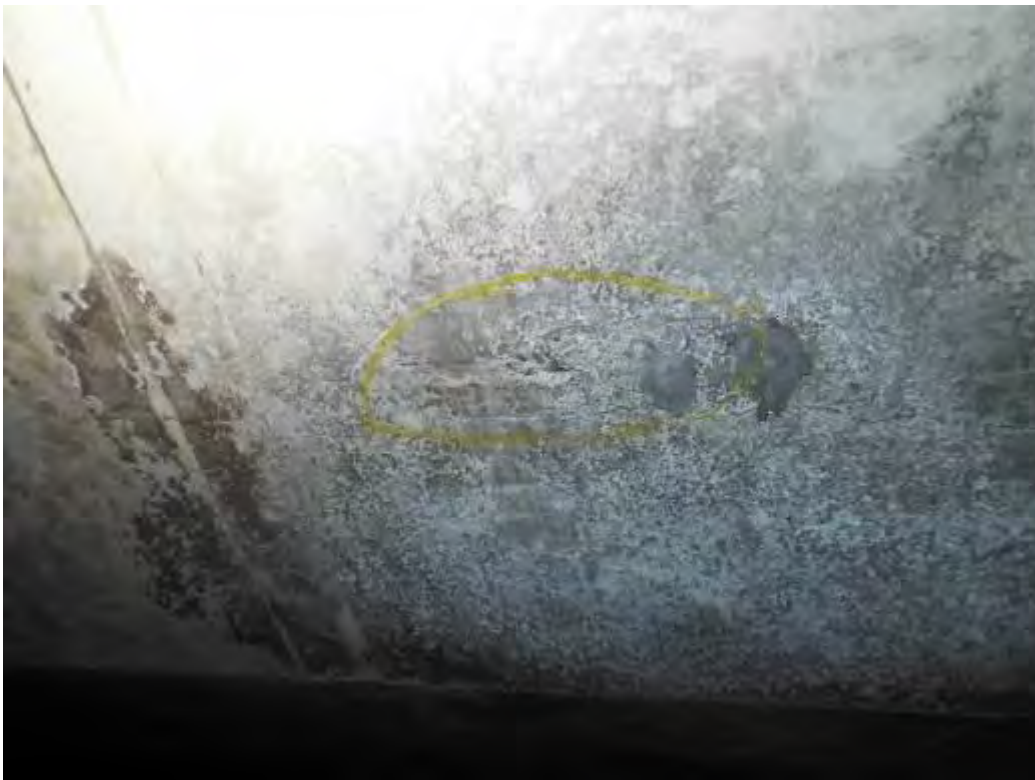
Photograph No.31 - Localised areas of spalled concrete on deck slab exposing reinforcement in span No3.
