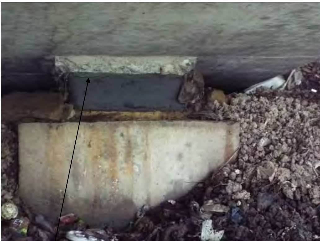
Photograph No.55 - Minor cracking to top of elastomeric pad on bearing No.2 at ESP 5. Detailed inspection restricted due to access beneath soffit and bearing plinths.
