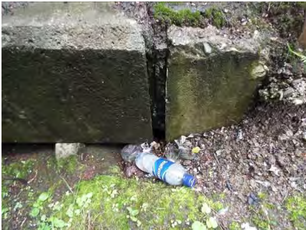
Photograph No.59 - Missing polysulphide sealant at both sides of ESP 5 on parapet fascia.
