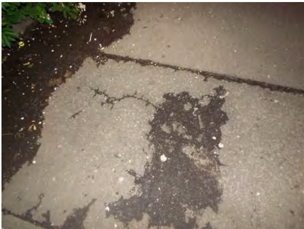
Photograph No.13 - (Typical) Cracks are evident in top layer of the surfacing.
