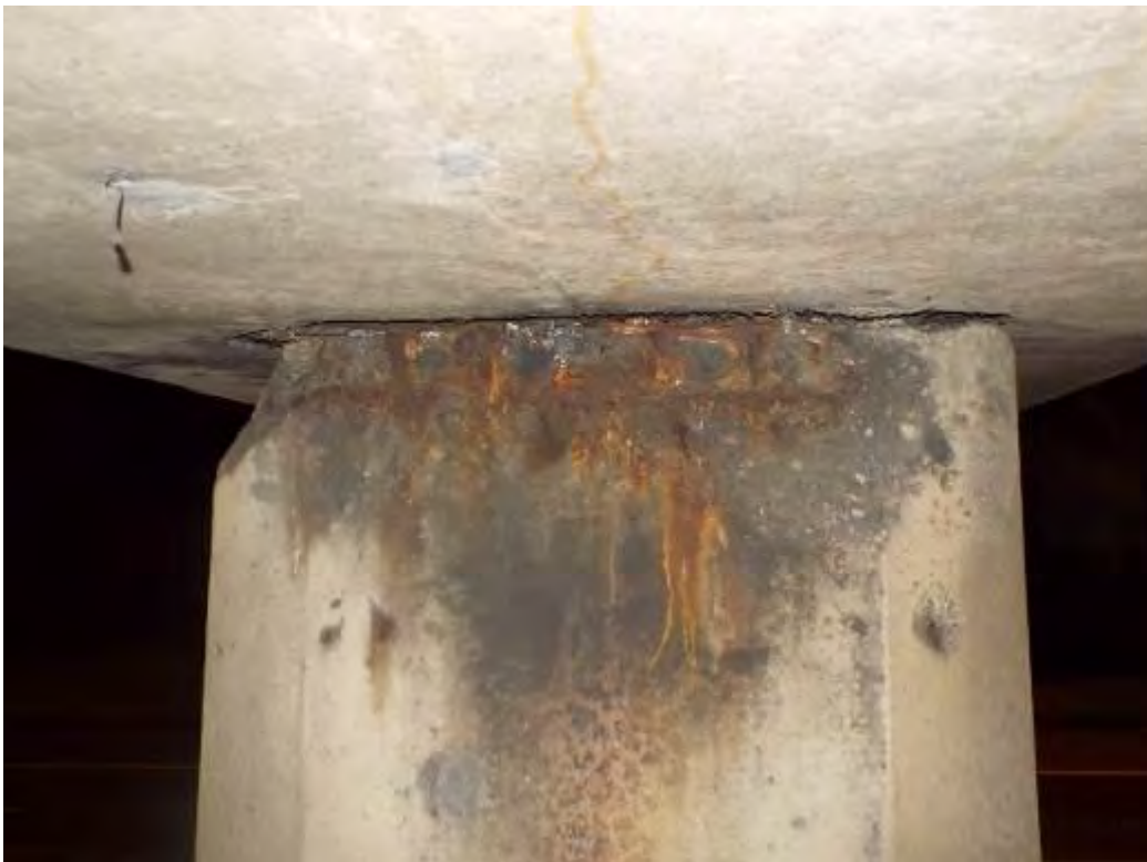
Photograph No.19 - Expansive corrosion of embedded reinforcement is resulting in rust staining at top of intermediate support No3 on uplink face.
