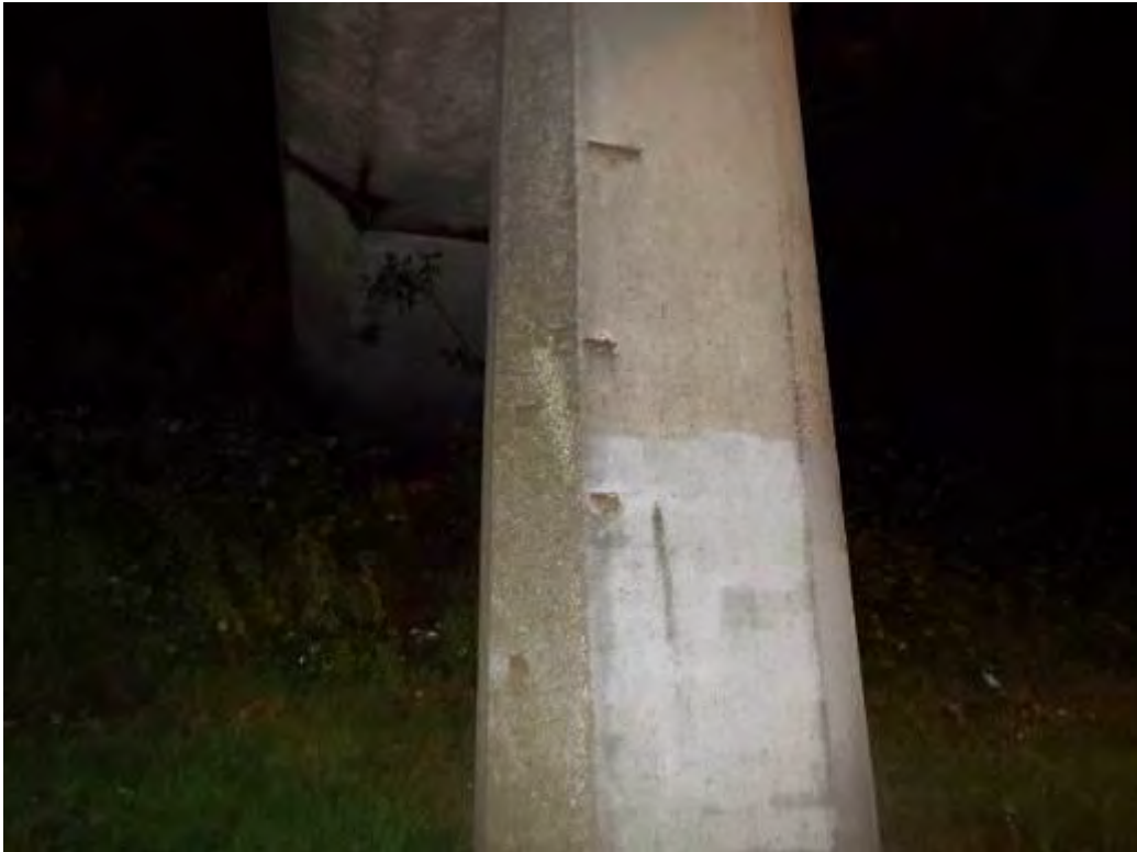
Photograph No.5 - Minor localised spalling exposing localised areas of reinforcement on ISP 2.
