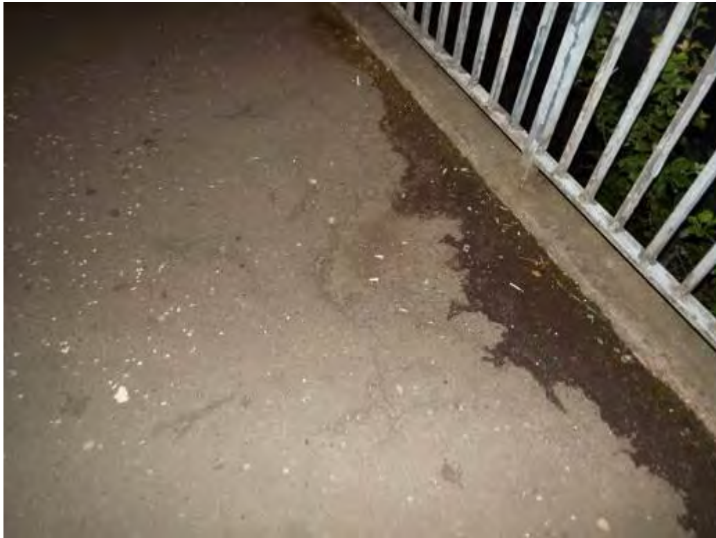
Photograph No.12 - (Typical) Footpath surfacing appears to have been treated with road salts / grit which may affect the condition of the concrete. Surfacing is ponding due to existing levels and lack of drainage outlets.
