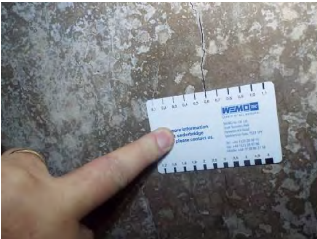
Photograph No.27 - Transverse cracking of reinforced concrete deck slab >0.6mm in places.
