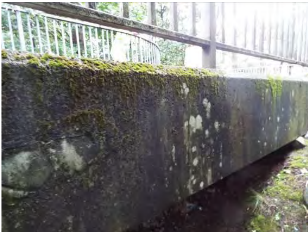
Photograph No.53 Moss growth on parapet upstand and fascia at both sides of span 4.
