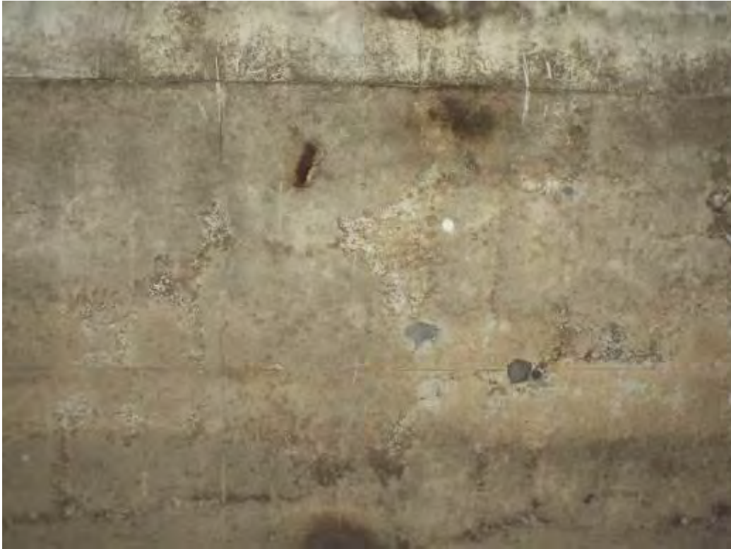
Photograph No.18 - Minor spall exposing reinforcement on soffit of deck slab at LHS.
