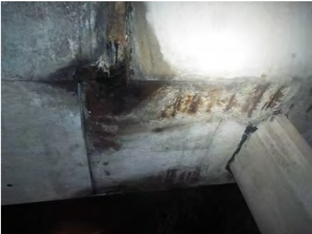
Photograph No.33 - Cracked / delaminated and spalled concrete on soffit and half joint at uplink side of span No3 on downlink side of intermediate support No4.
