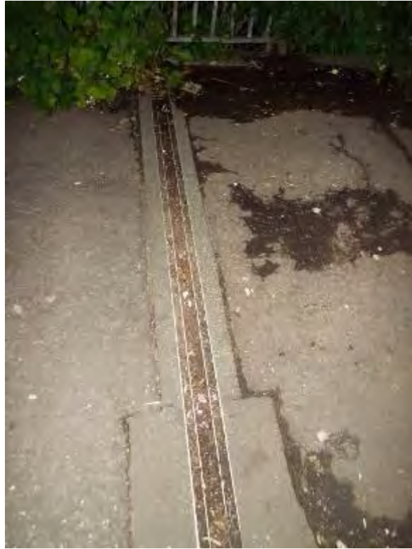
Photograph No.6 - Expansion joint rubber inserts at end support No1 in span No1 blocked with debris.
