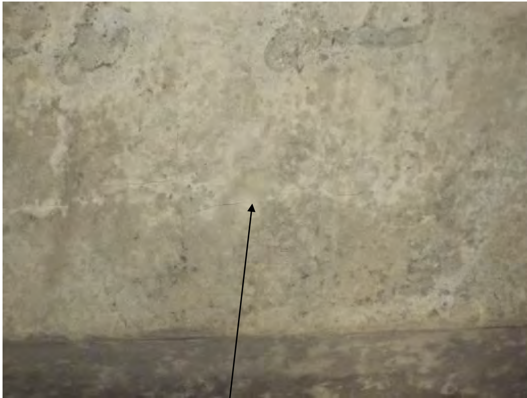
Photograph No.28 - Longitudinal cracking of reinforced concrete deck slab >0.3mm in places.
