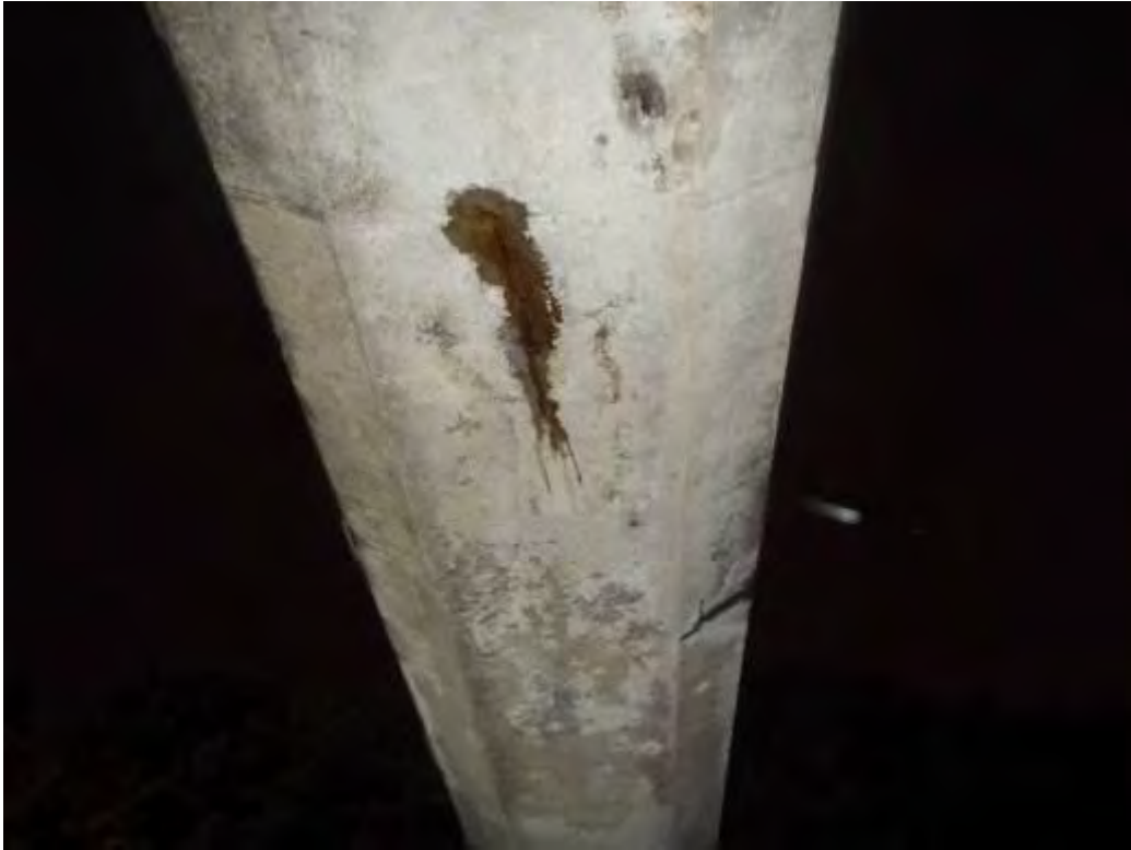
Photograph No.42 -The soffit of the structure shows signs of seepage in span 3.
