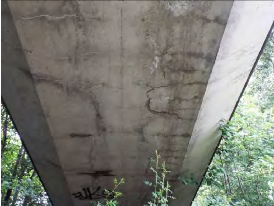
Photograph No.52 - Expansive corrosion of embedded reinforcement resulting in delamination and spalling exposing reinforcement on the soffit of the RC slab.
