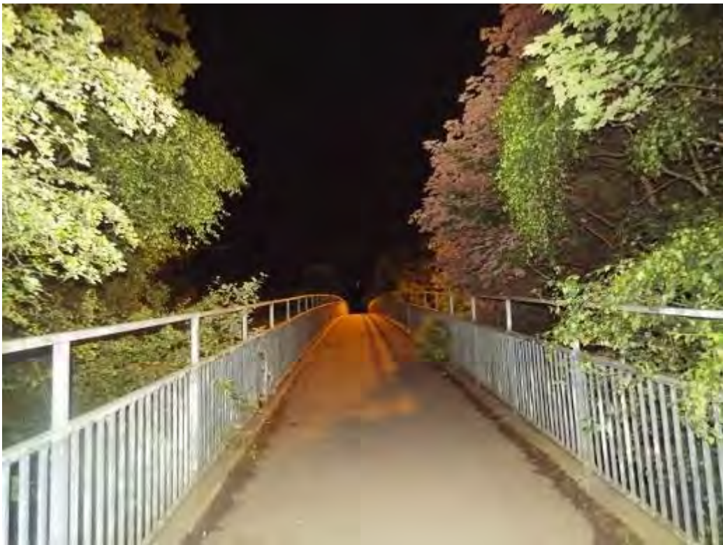
Photograph No.61 - (Typical) Minor vegetation growth at both sides of the footpath.
