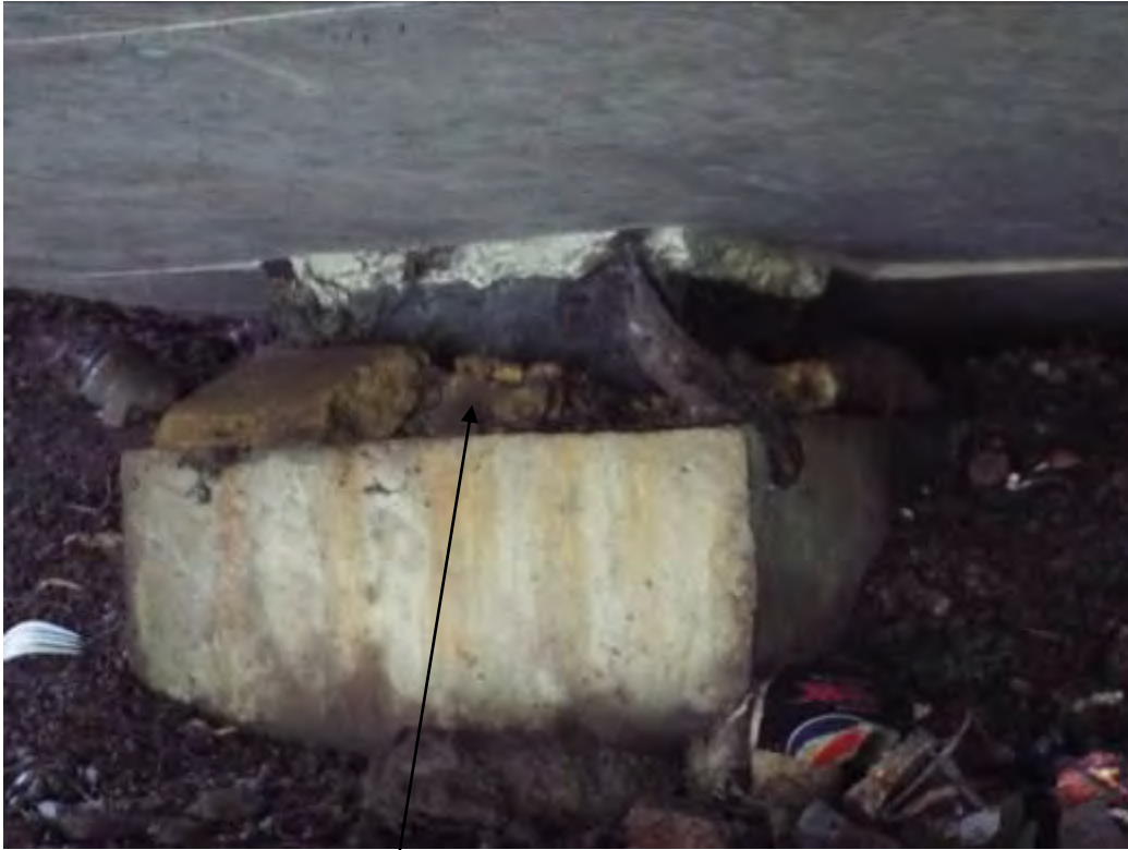
Photograph No.56 - Minor spalling of the mortar base around the bearings at ESP 5.
