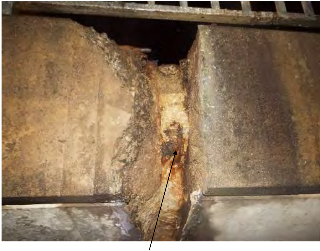
Photograph No.40 - Moderate spalling exposing mortar cap to post tensioned anchor block at uplink half joint RHS.
