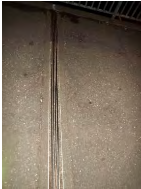
Photograph No.7 - Expansion joint rubber inserts at Half joint in span No1 blocked with debris.
