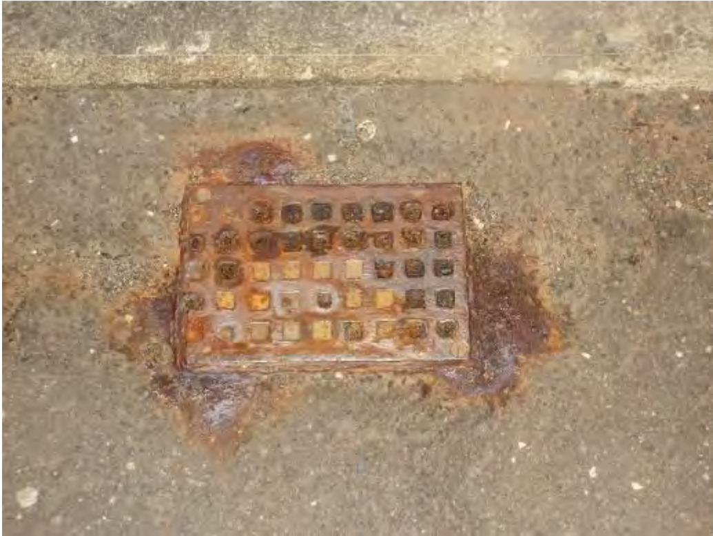
Photograph No.22 - Gully grating cover completely blocked preventing water from entering drainage system.
