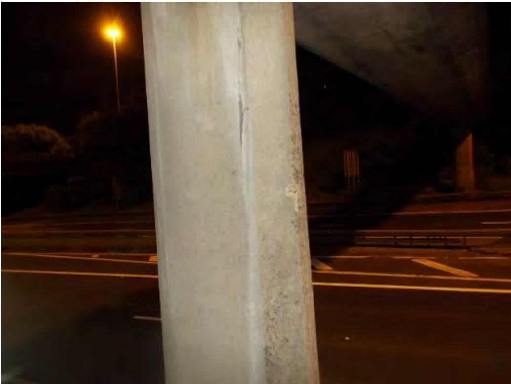
Photograph No.21 - Minor impact damage on ISP 3 at LHS.
