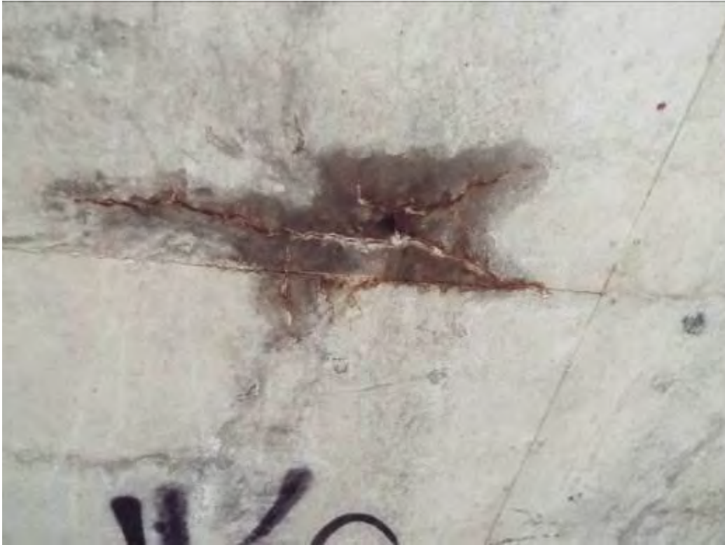
Photograph No.48 - Transverse cracking with leaching on reinforced concrete deck soffit >0.3mm in places.
