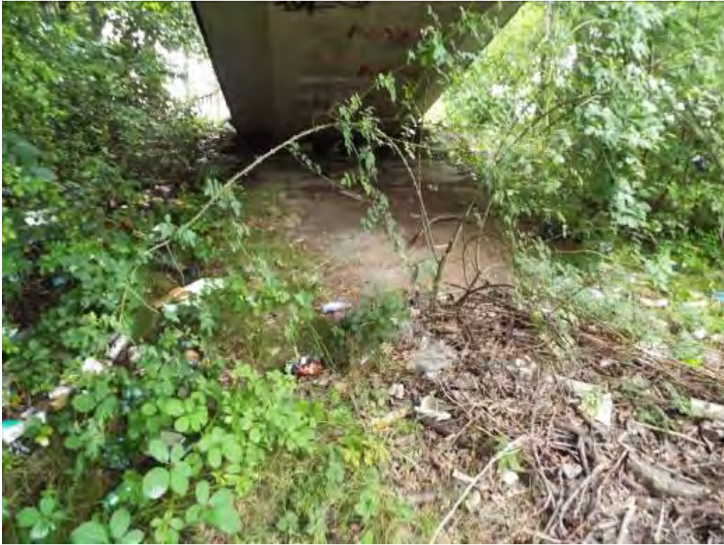
Photograph No.62 - Vegetation growth and build of litter making area unsightly on embankment in span 4.
