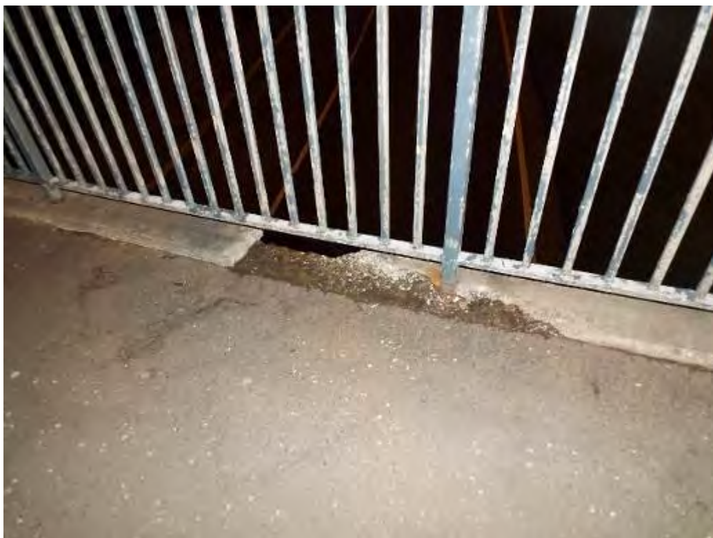
Photograph No.37 - Parapet upstand and showing evidence of scaling from frost damage and salt attack exposing aggregate of concrete in places.
