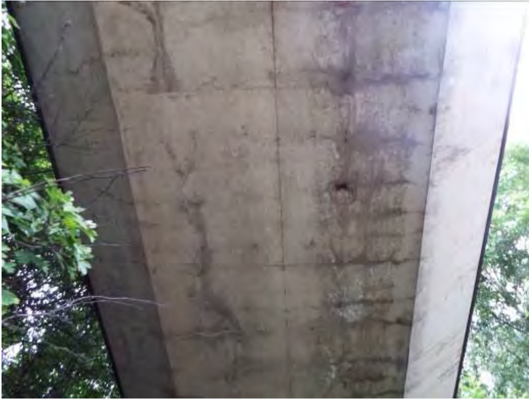
Photograph No.50 - Longitudinal and transverse cracking on reinforced concrete deck slab and soffit >0.3mm in places.
