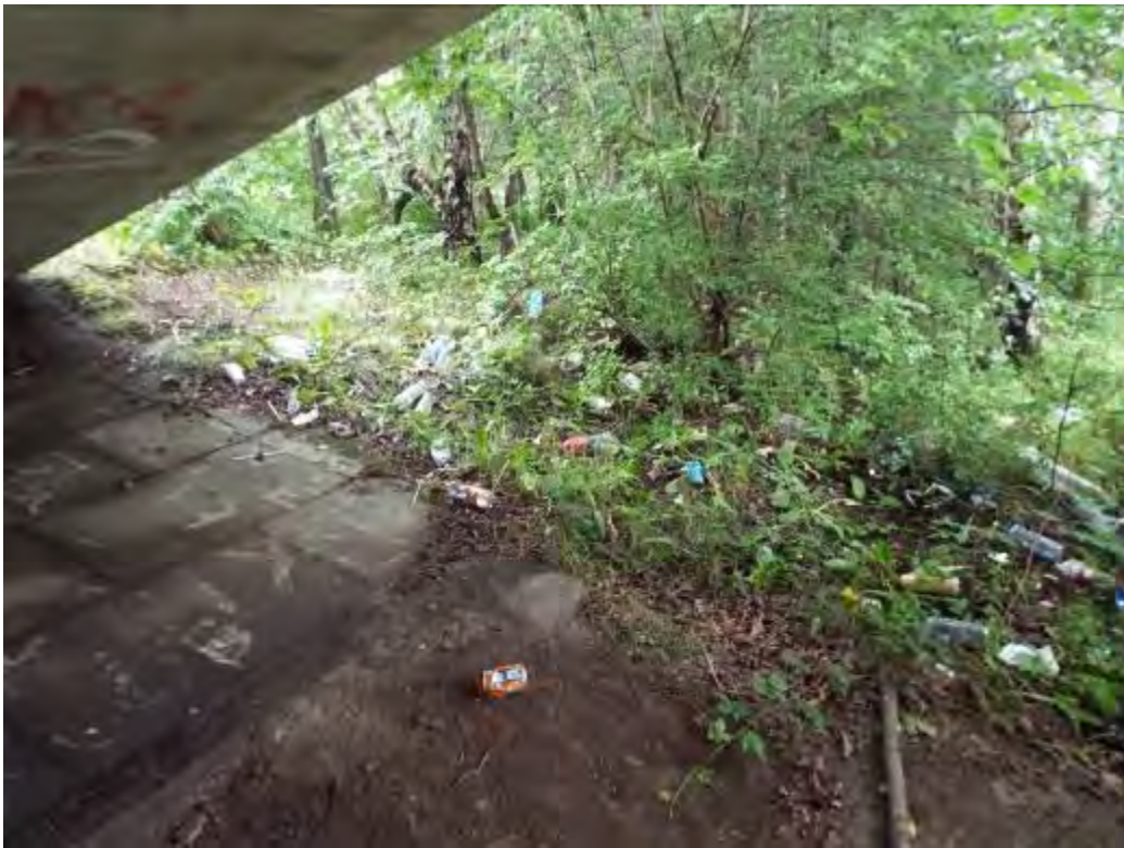
Photograph No.63 - Vegetation growth and build of litter making area unsightly on embankment in span 4.
