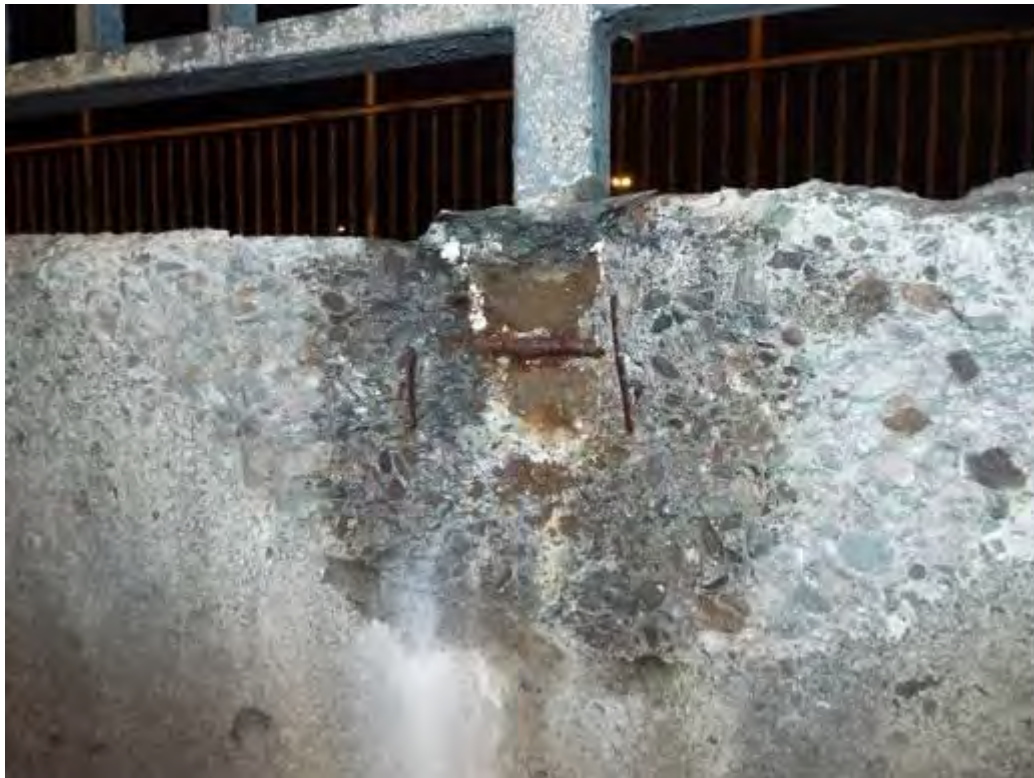
Photograph No.17 - Moderate localised spall where handrail parapet is recessed into concrete of parapet upstand. At LHS above lane 2 of M8 westbound.
