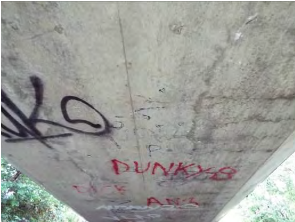
Photograph No.49 - Longitudinal cracking on reinforced concrete deck soffit >0.3mm in places.
