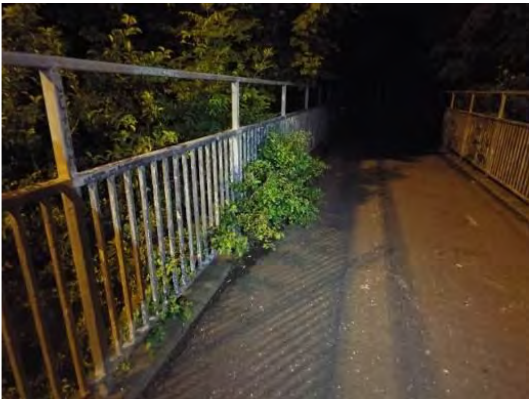
Photograph No.65 - Vegetation growth encroaching on RHS parapet rail in span 4.
