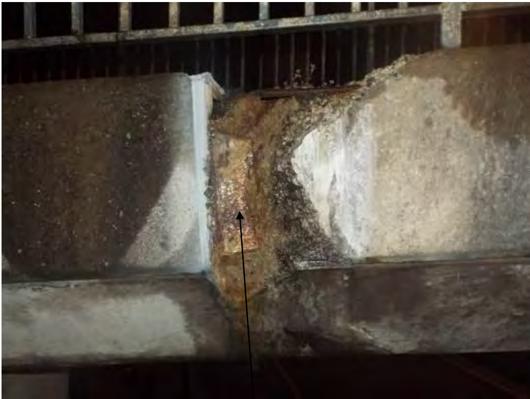
Photograph No.39 - Moderate spalling exposing mortar cap to post tensioned anchor block at uplink half joint LHS.
