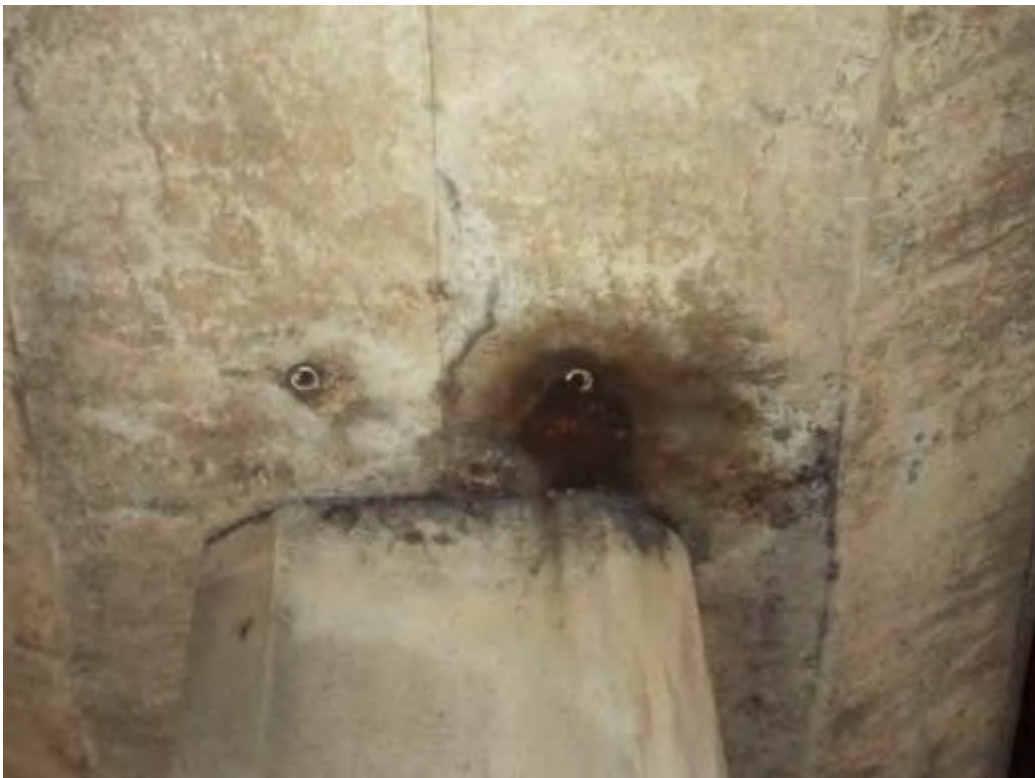
Photograph No.23 - Deck dripper blocked causing staining on Span 2 soffit adjacent ISP 3 downlink face.
