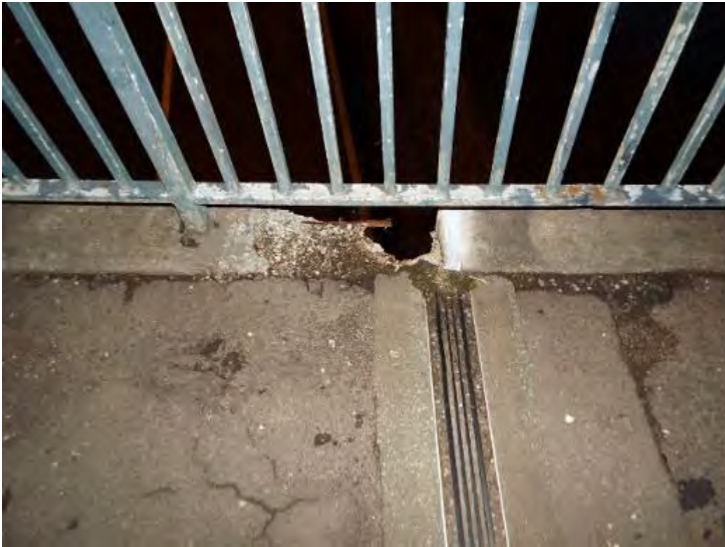
Photograph No.38 - Parapet upstand and showing evidence of scaling from frost damage and salt attack exposing aggregate of concrete in places at half joints which is providing path for water to saturate joint interface below.
