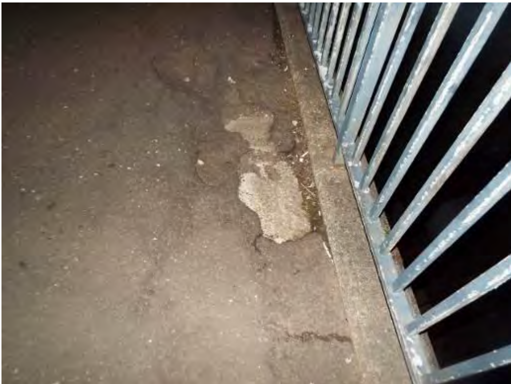
Photograph No.47 - Footpath surfacing is breaking up exposing localised areas of concrete. Waterproofing is not present at localised areas due to weathering and foot traffic on the structure.
