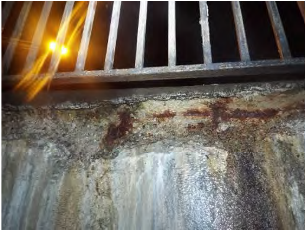
Photograph No.36 - Parapet upstand and showing evidence of scaling from frost damage and salt attack exposing aggregate of concrete in places. Also localised spalls on concrete of parapet fascia.
