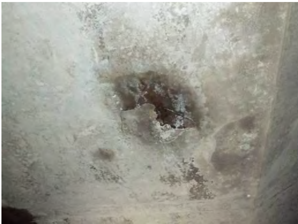
Photograph No.29 - Localised areas of spalled concrete on soffit and exposing reinforcement in span No3.
