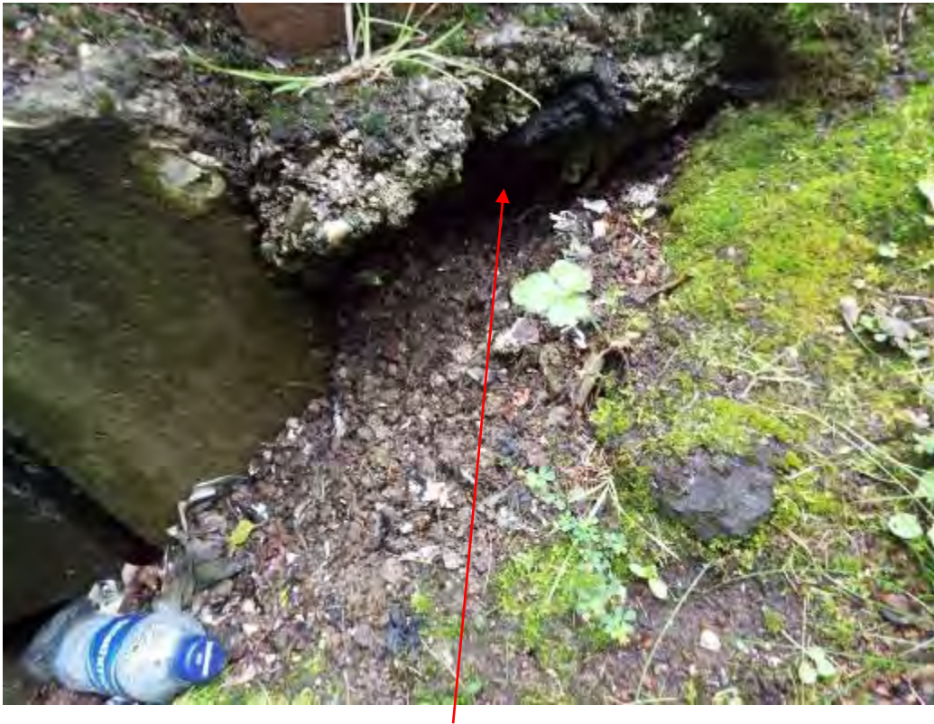
Photograph No.64 - Minor undermining of parapet beam at uplink RHS of ESP 5.
