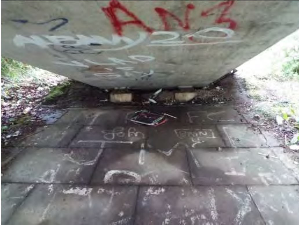
Photograph No.54 - Due to geometry of soffit of the structure where it intersects with the revetment the bankseat abutment is hidden from view at end support No5.
