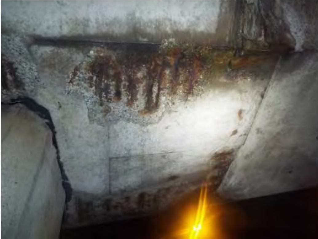
Photograph No.32 - Cracked / delaminated and spalled concrete on soffit at half joint uplink side of span No3 on downlink side of intermediate support No4.
