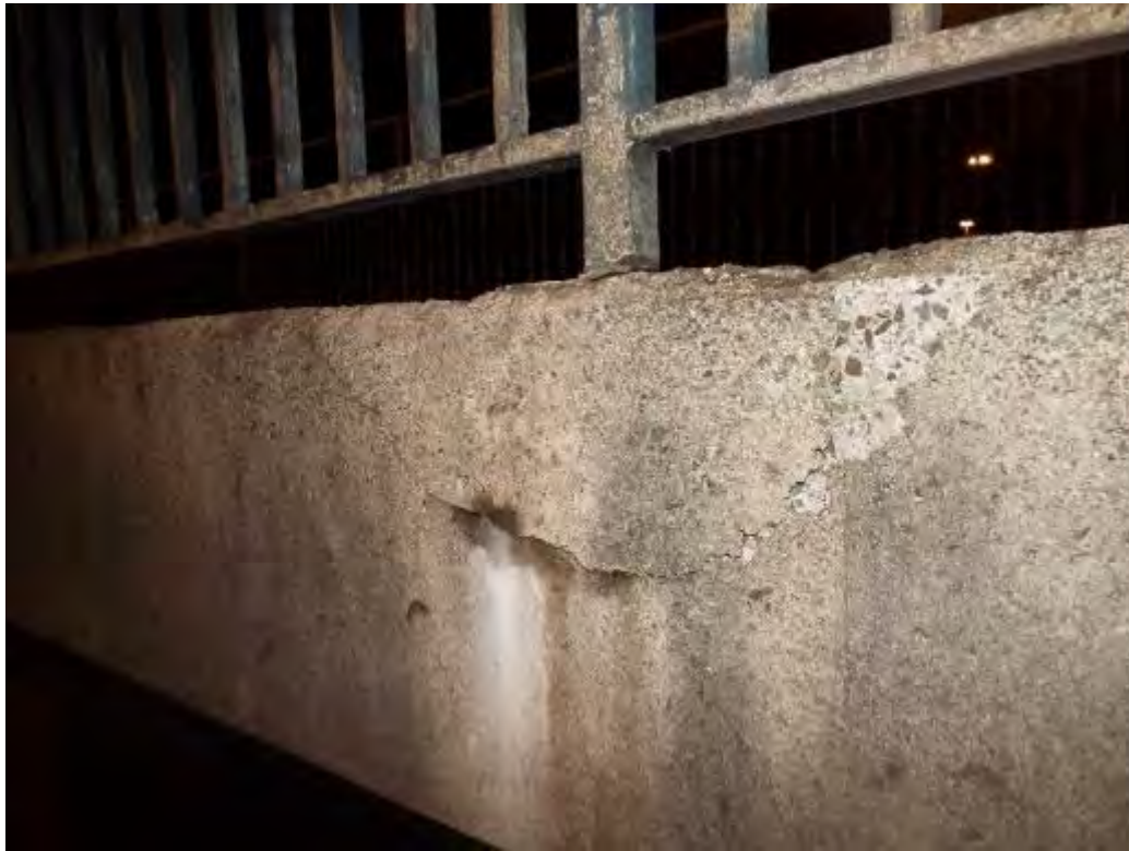
Photograph No.16 - Moderate localised spall where handrail parapet is recessed into concrete of parapet upstand. At LHS above lane 2 of M8 westbound.
