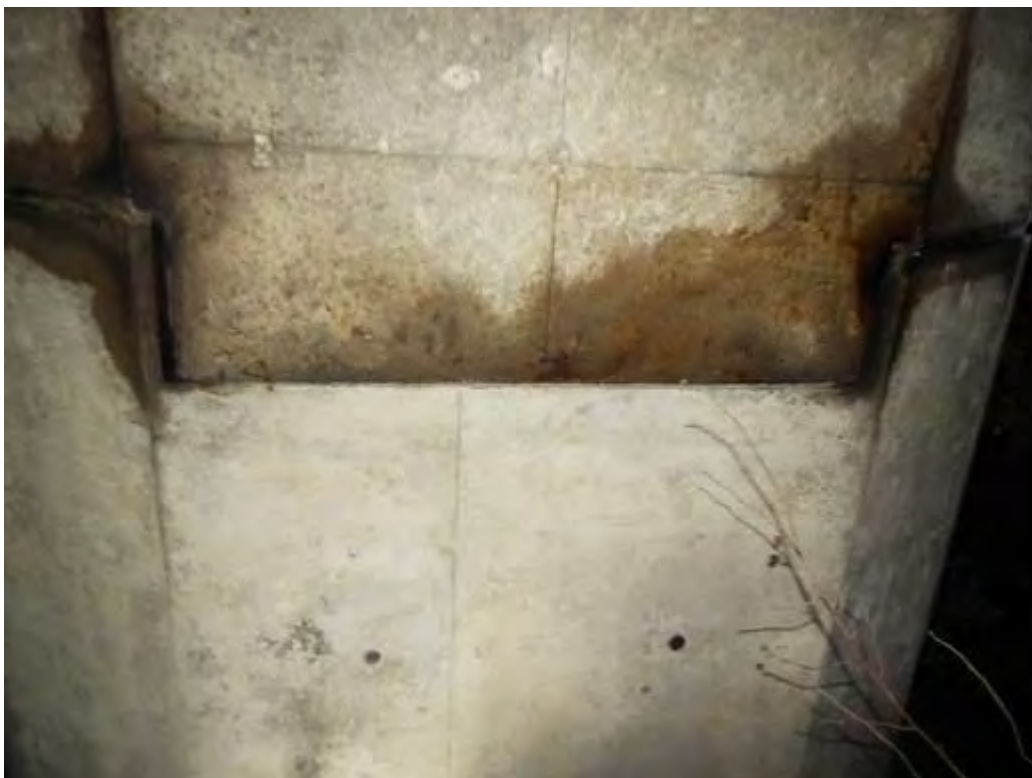
Photograph No.3 - Staining at half joint as a result of seepage through de-bonding sealant at parapet upstand joint above in span 1.
