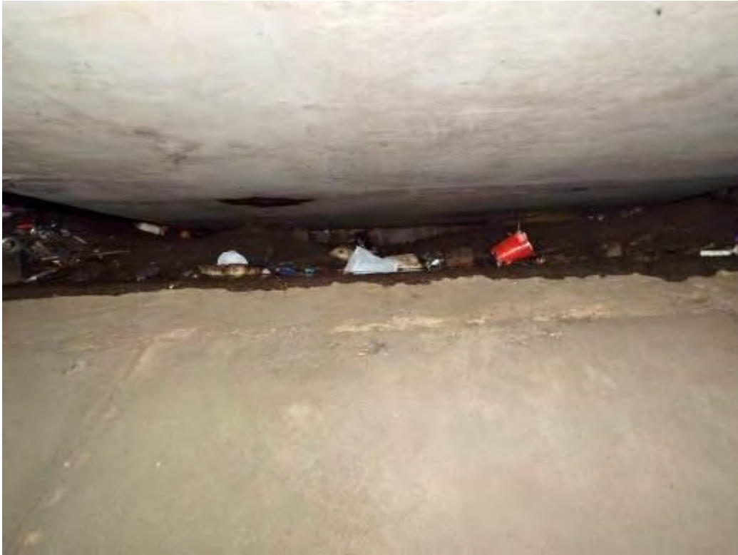
Photograph No.4 - Leaching and dampness on exposed area of bank seat curtain wall at ESP 1. Access to inspect area difficult due to access beneath soffit.
