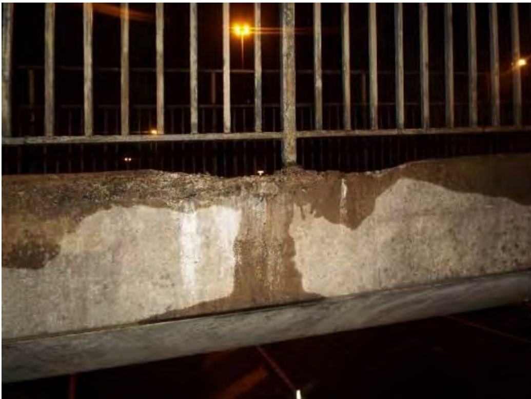
Photograph No.35 - Parapet upstand and showing evidence of scaling from frost damage and salt attack exposing aggregate of concrete in places.
