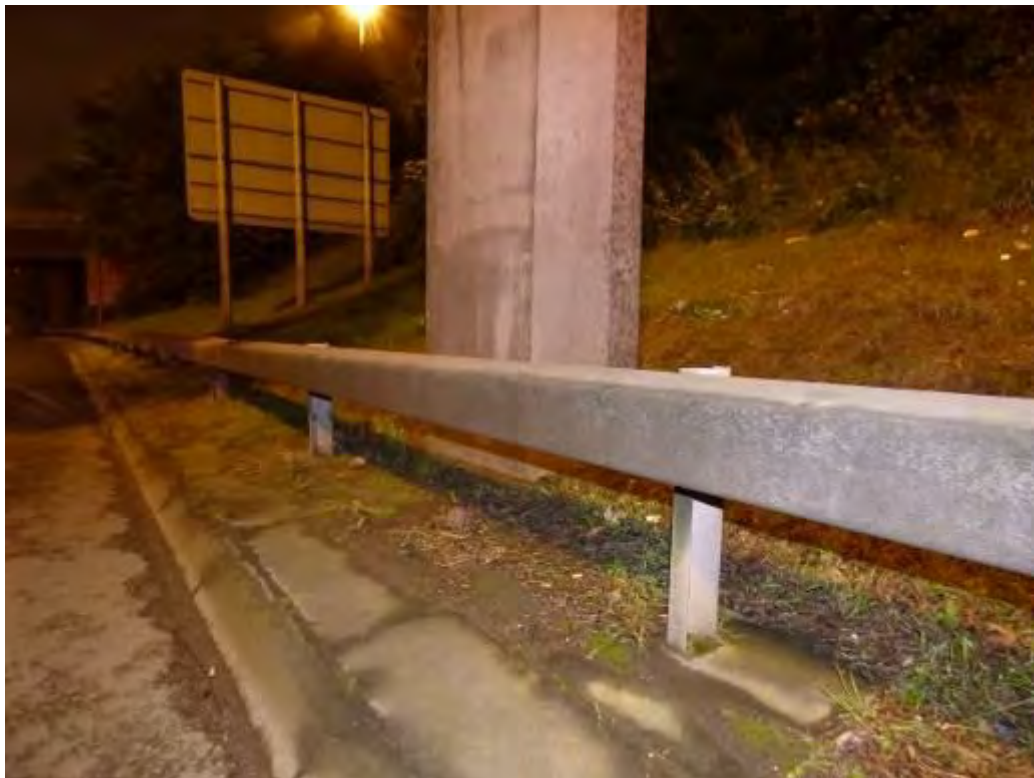
Photograph No.25 - Safety barrier currently single height OBB protecting slender pier at intermediate support No2. Due to increase traffic from new M74 on secondary carriageway barrier height / containment should be reviewed.
