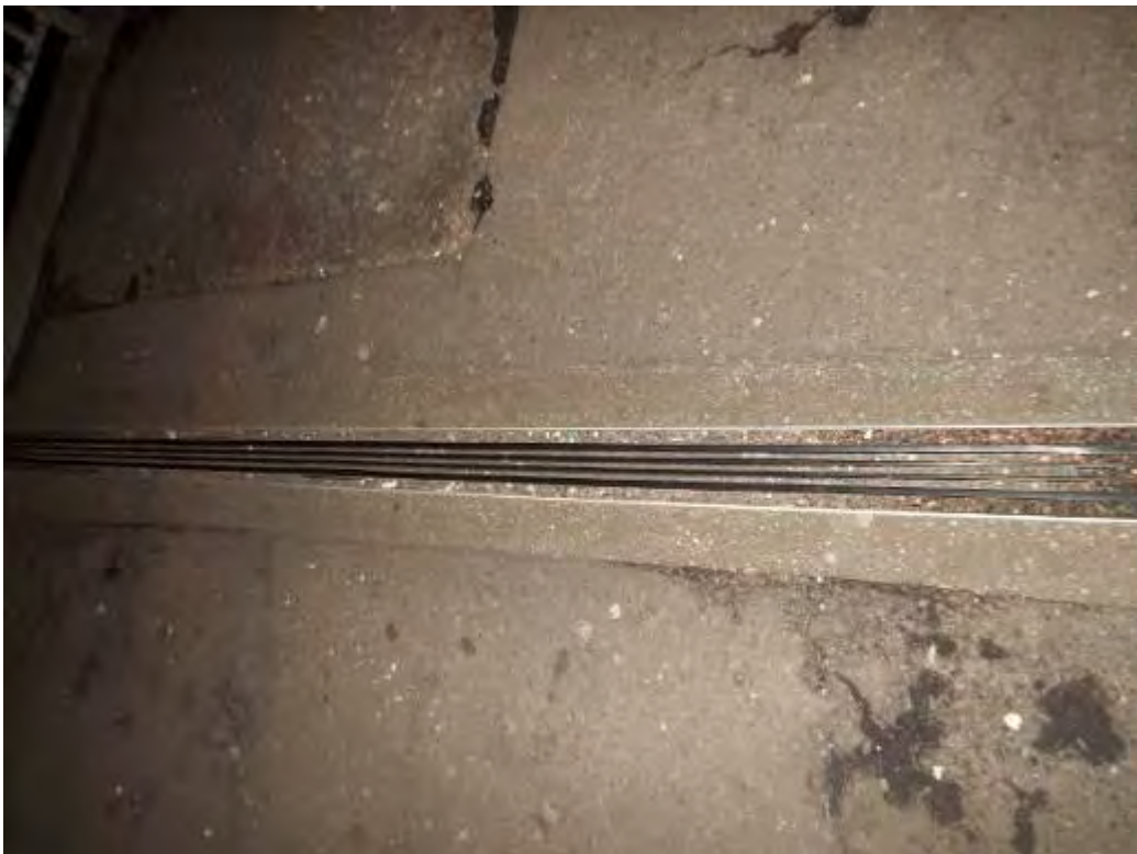
Photograph No.43 - Expansion joint rubber inserts at Half joints in span No3 blocked with debris.
