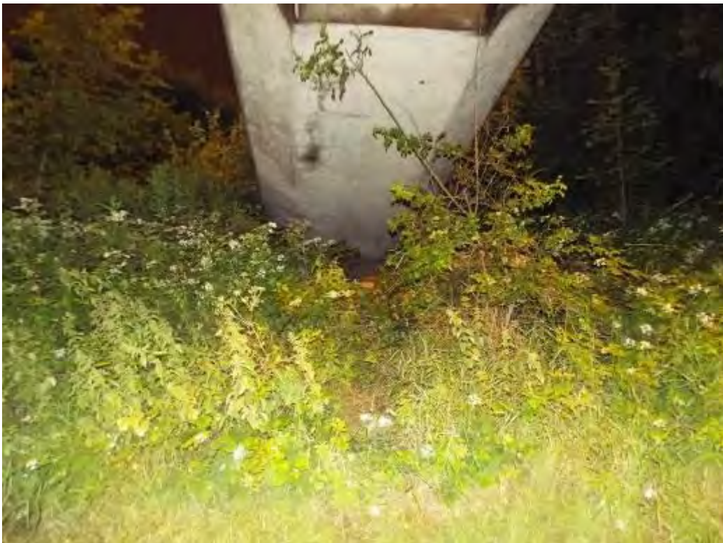
Photograph No.15 - Moderate vegetation growth on embankment in span 1.
