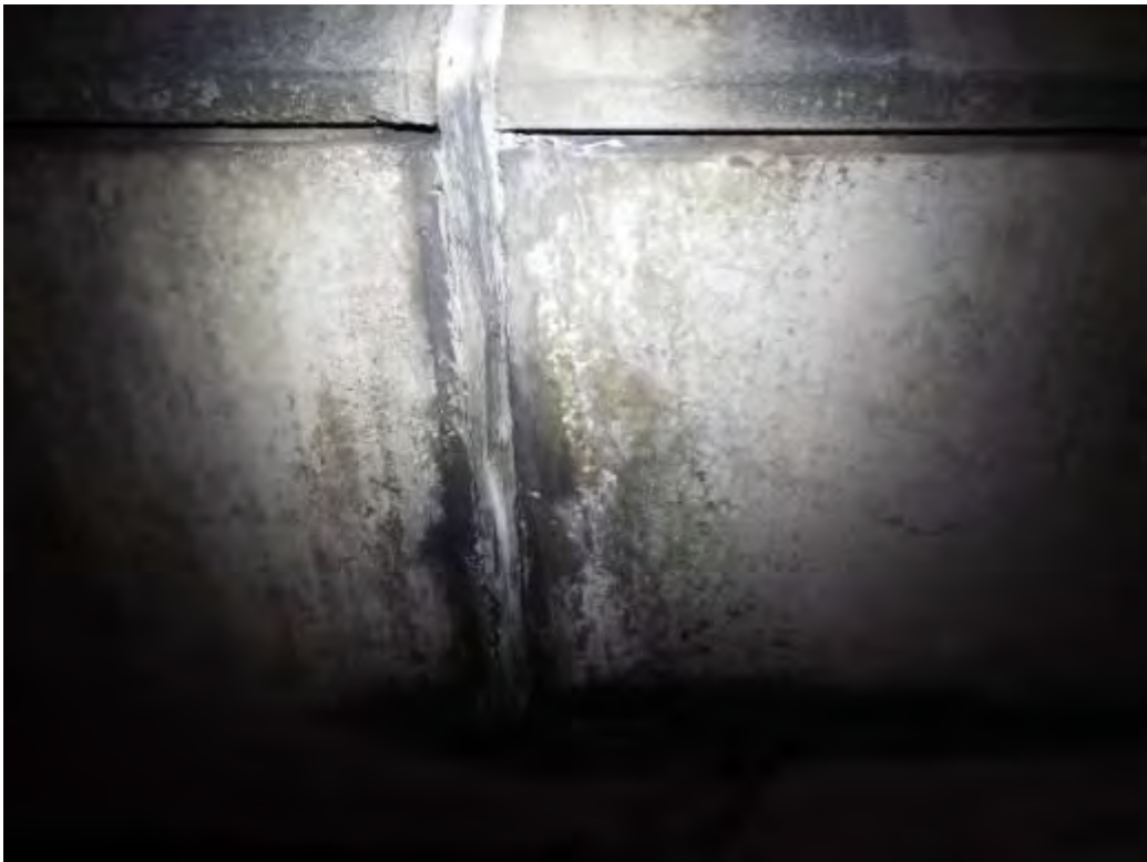
Photograph No.45 - Polysulphide sealant de bonded at both sides of half joint in span 3.
