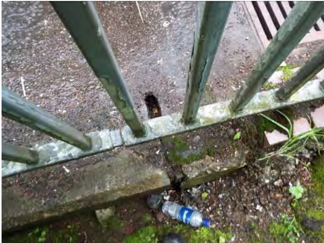
Photograph No.58 - Missing polysulphide sealant at both sides of ESP 5 parapet upstand.
