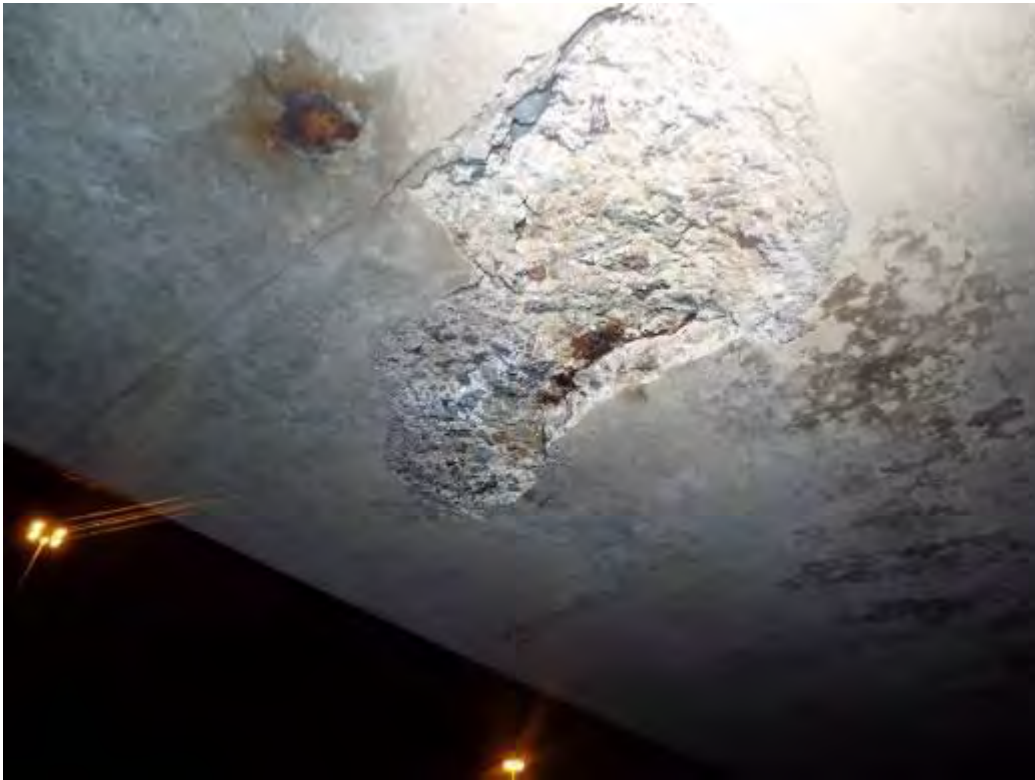
Photograph No.30 - Localised areas of spalled concrete on soffit exposing reinforcement in span No3.
