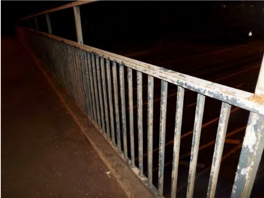
Photograph No.10 - (Typical) Existing paint system is beyond its useful life span. All paint coats failed.
