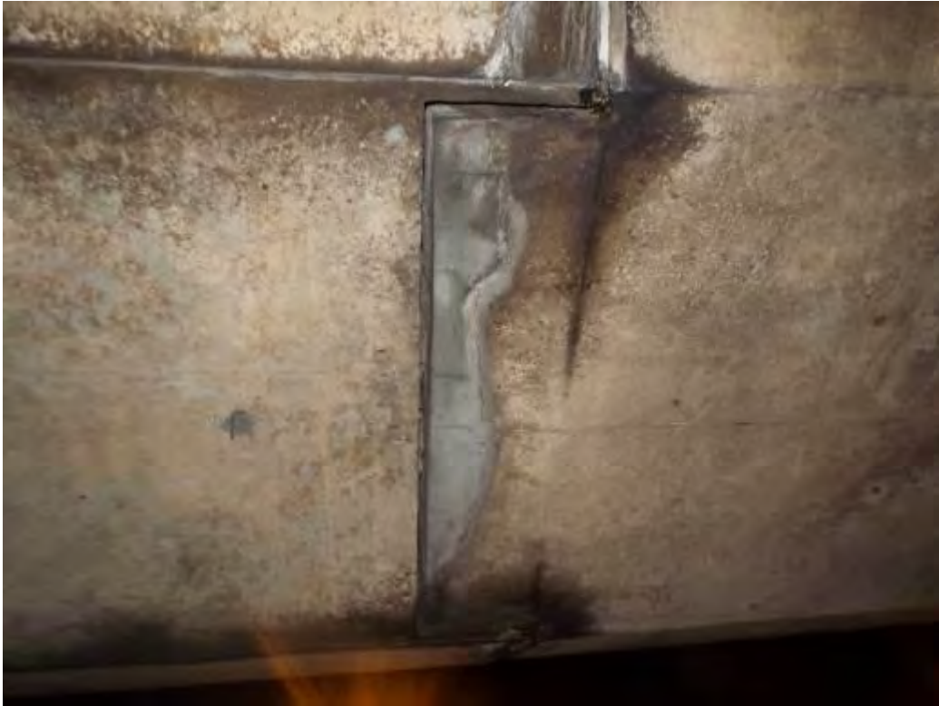
Photograph No.44 - Minor leakage through expansion joint rubber insert at both half joints in span 3 and through polysulphide joint in the parapet upstands at the half joints.
