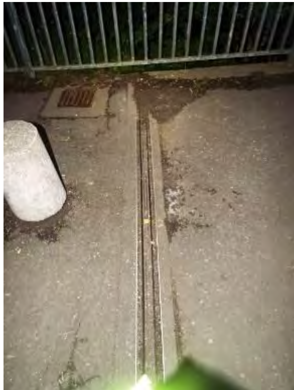
Photograph No.57 - Expansion joint rubber inserts at end support No5 joint in span No4 blocked with debris.
