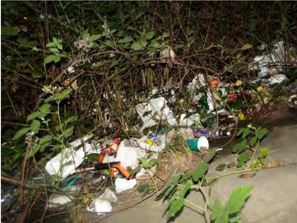
Photograph No.14 - Debris and build of litter making area unsightly on revetment in span 1.
