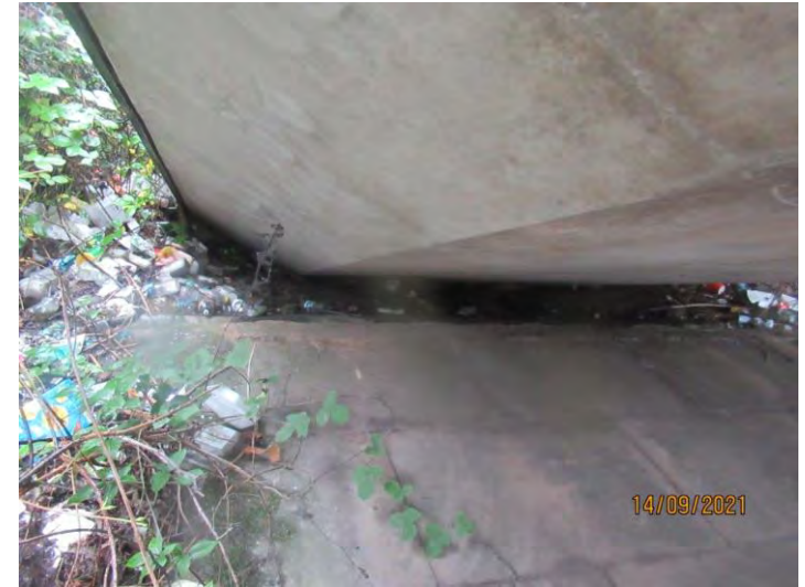
Photo 2 - Rubbish and debris on ES1 bearing shelf
