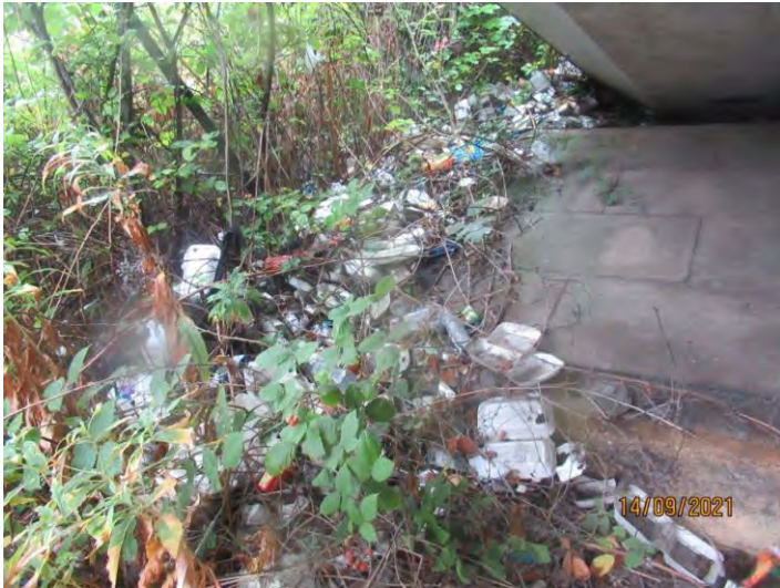
Photo 5 – Rubbish and debris on revetments
