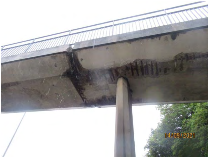
Photo 11 – Spalling on soffit
