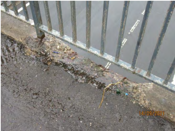
Photo 7 – Spalling on parapet edge beam
