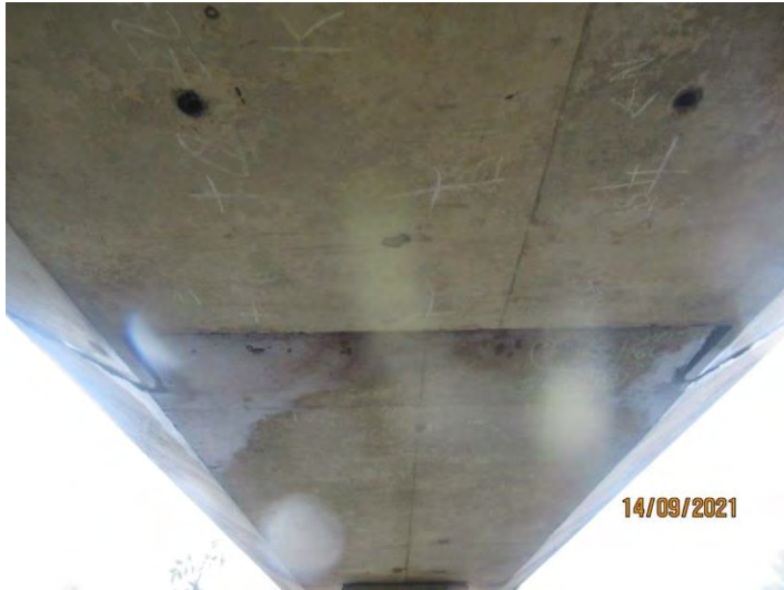
Photo 1 – Cracking on soffit
