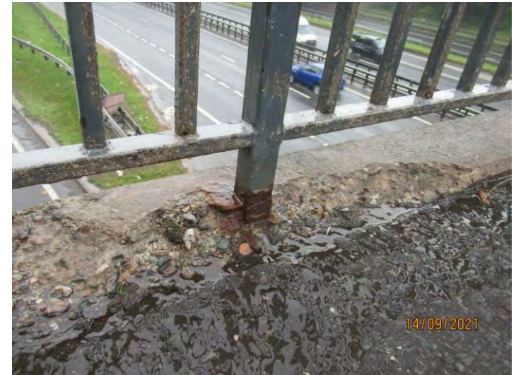
Photo 4 – Failed protective paintwork on parapets.
