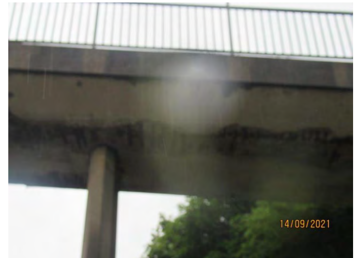
Photo 8 – Expansive corrosion at top of piers
