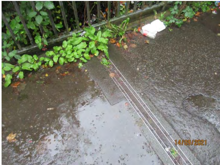
Photo 3 – Joints full of debris
