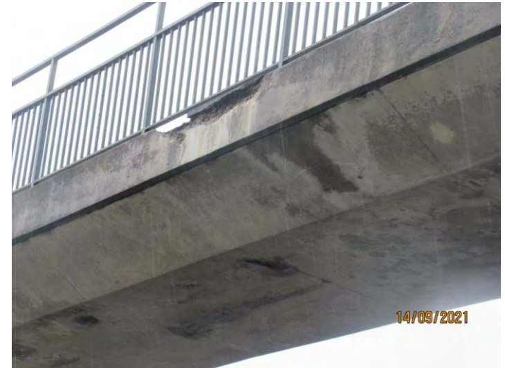
Photo 10 – Spalling to parapet edge beam
