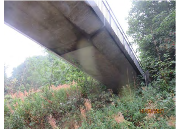
Photo 6 – Vegetation growth on embankments
