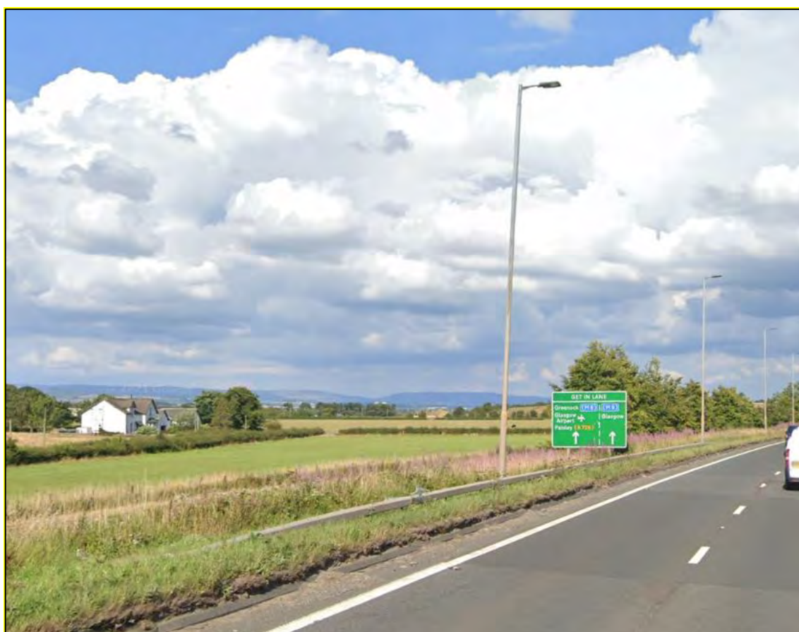
Figure 3-2 – A737 Mainline Northbound Verge Safe System Defects
