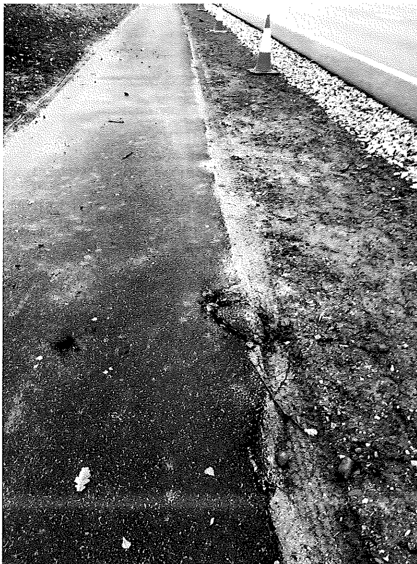
Problem 3.8 – Cracked Surface at Ch. 1060
