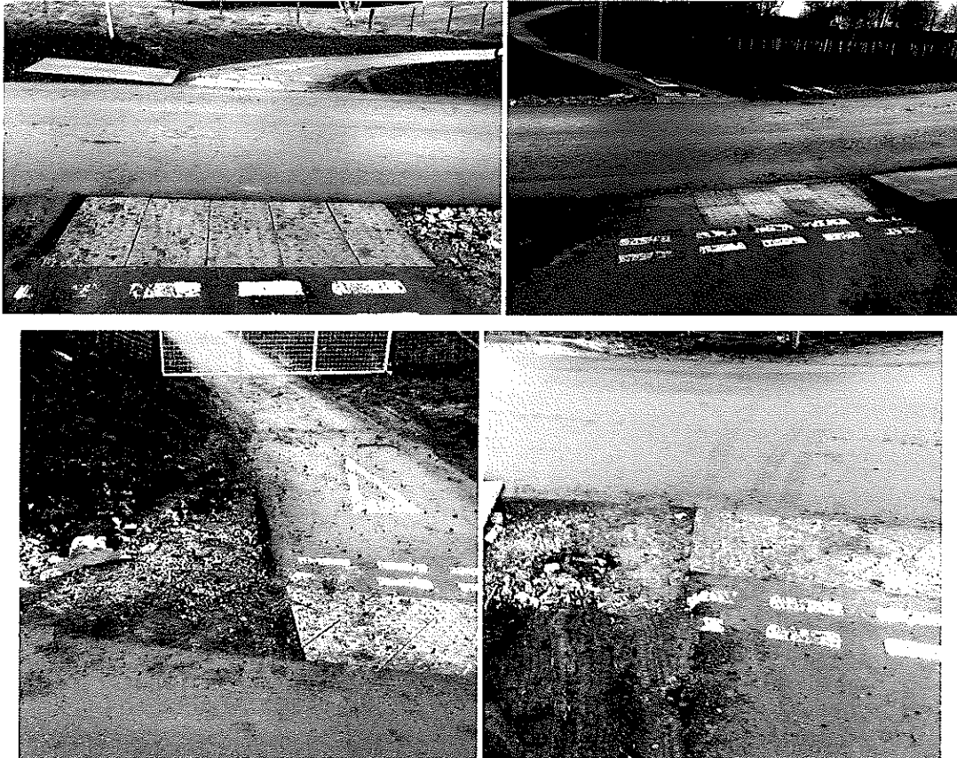
Problem 3.17 – Examples of Unfinished Works Around Tactile Paving
