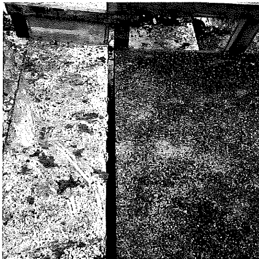
Problem 3.11 – Gap in NMU Watercourse Crossing Bridge
