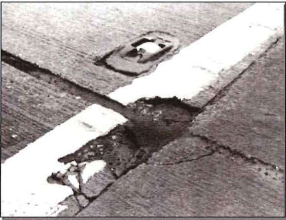
DSPL Deep spalling at joints
