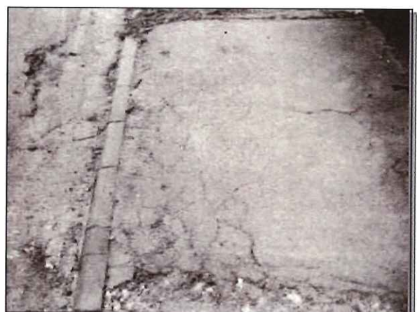
BECK Bituminous Surfacing – Extensive Cracking
