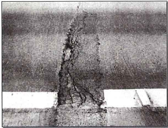
RFAL Failed Repair
