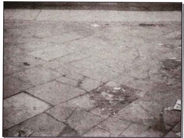
SLCK Slab Cracking
