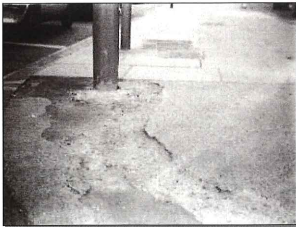
RLMT Trench RI – loss of material
