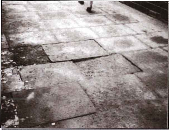
SLPF Slab profile – uneven/trips
