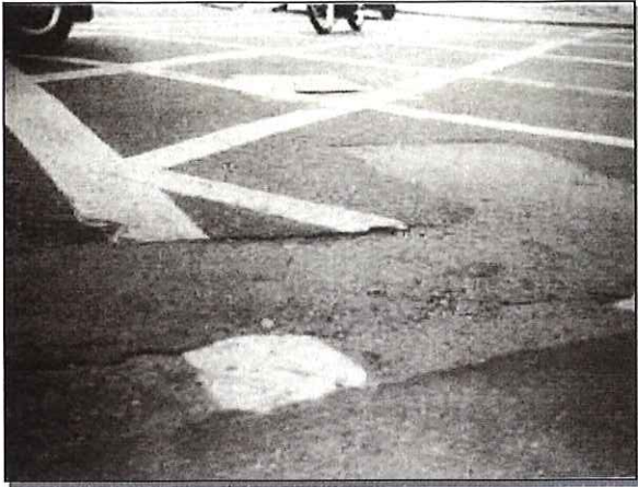
TLMT Trench RI - loss of material
