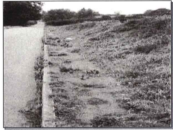
OVGV Overgrown by vegetation
