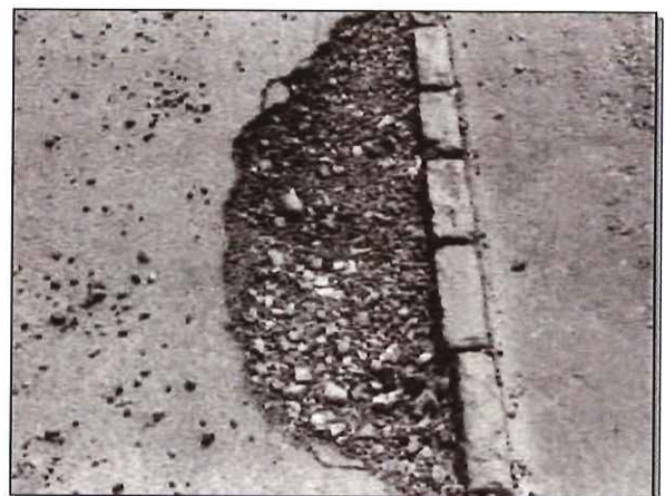
BPOT Bituminous surfacing – potholes
