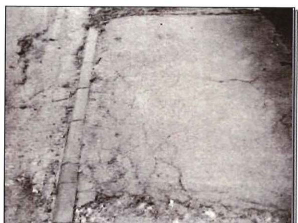
BECK Bituminous Surfacing – Extensive Cracking
