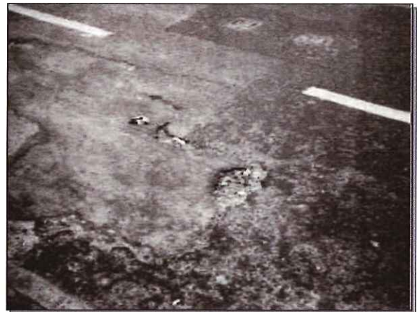
PLMT Patch – loss of material
