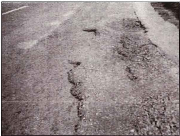
PDLV Patch – difference in level
