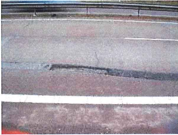
OVSD Failed overbanding / sealed cracks
