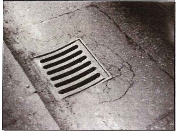
CKIR Cracking around ironwork
