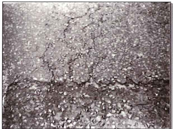
TACK Trench RI – adjacent cracking
