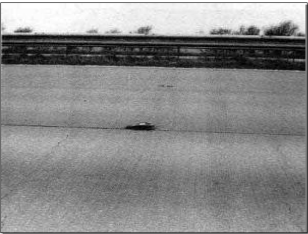
MISC Missing Catseye
