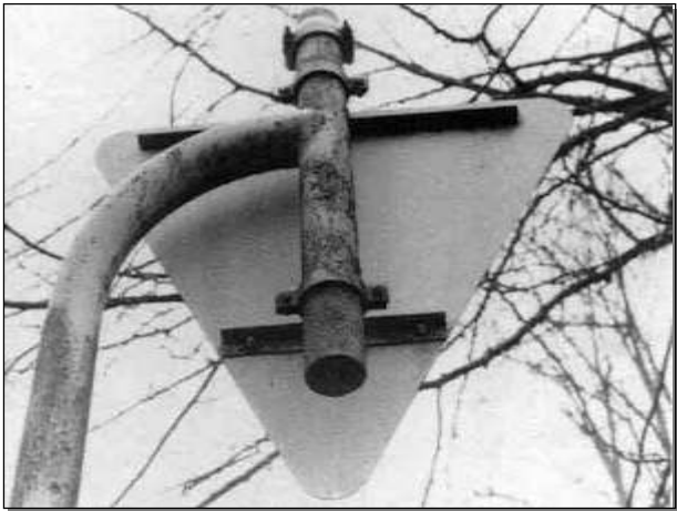
SFCO Surface corrosion
