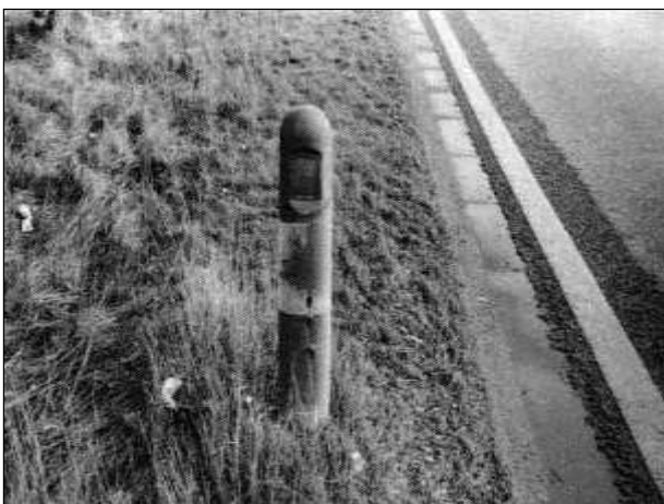
COPT Physical condition of post
