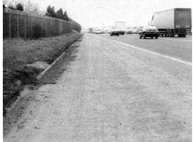
MUCK Excessive Muck
