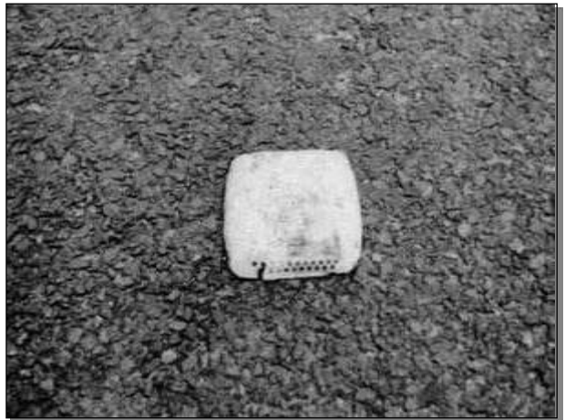
DAMS Damaged stud
