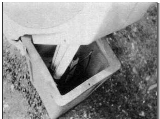
EXPW Exposed wiring
