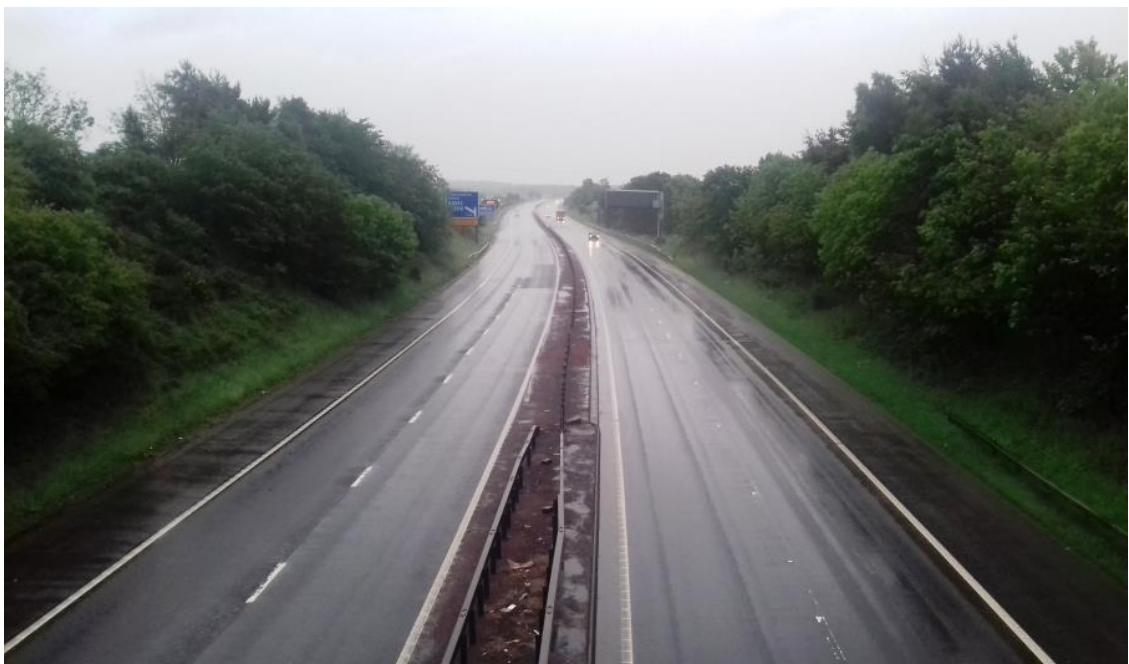
Junction 2 looking SB – Photo shows surface water flowing across the carriageway from the Northbound Hardshoulder.
