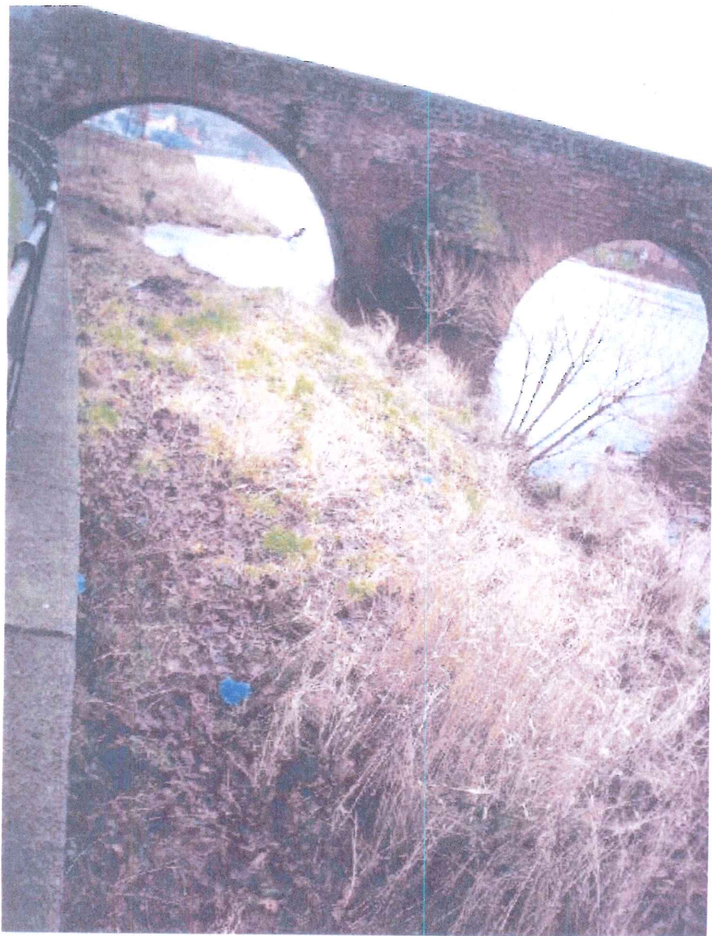
AREA OF SILT IN WINTER LOCATION DEVBAGINNA BRIDGE
