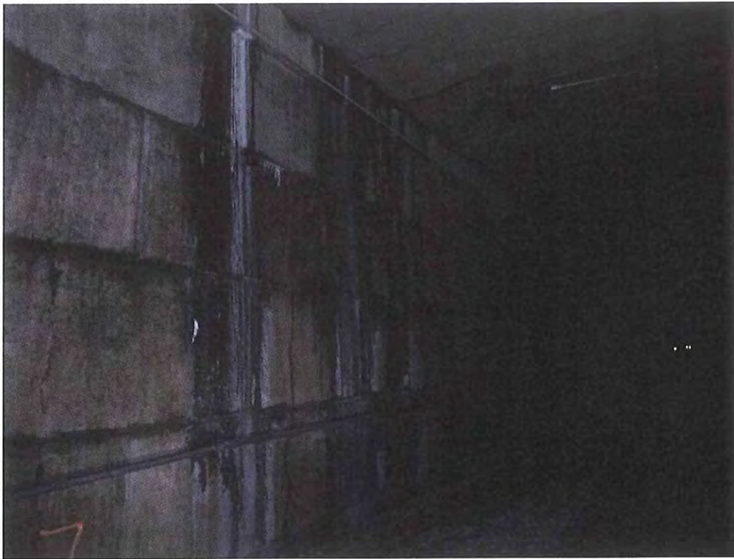
Photo D4 – DEFECT: - Historic water staining of abutments
