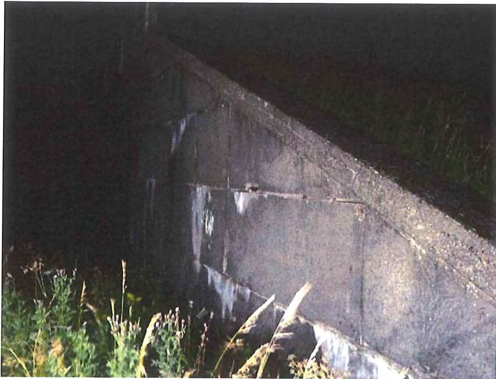
Photo G9 -RHS Uplink WINGWALLS
