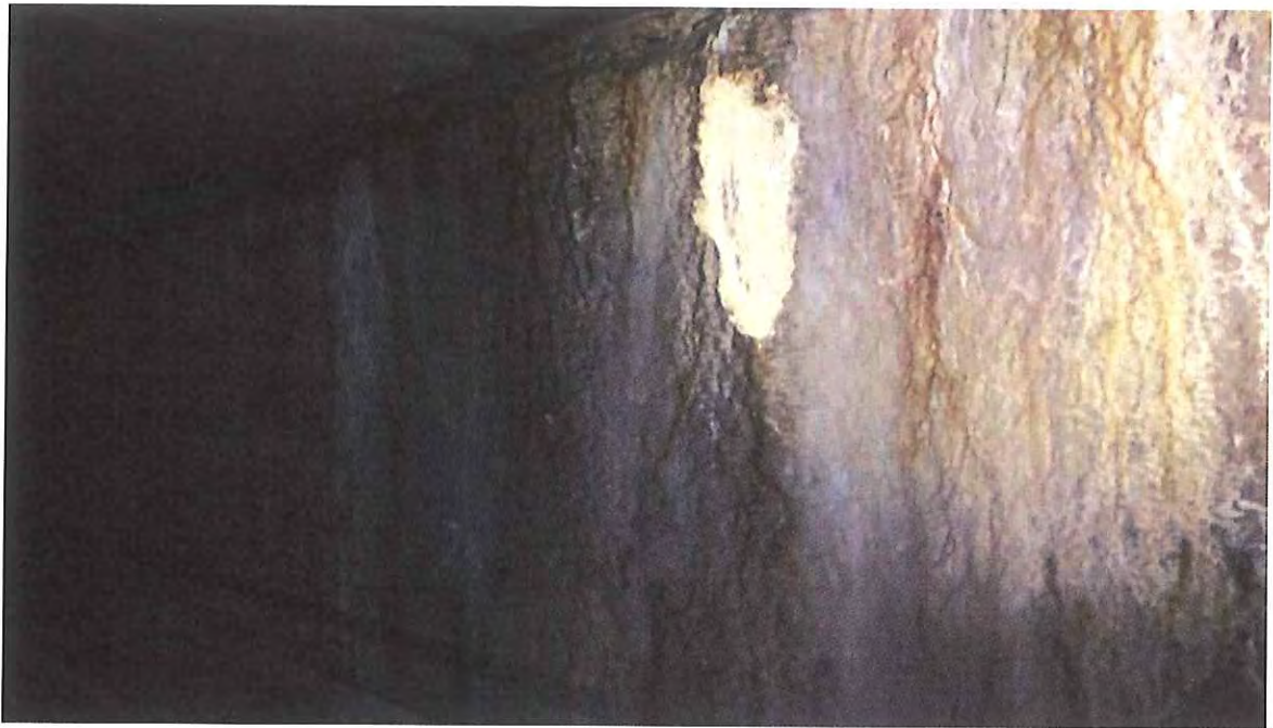
Photo D10 – DEFECT: - Efflorescence on Abutment
