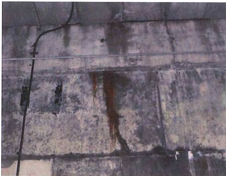
Photo D7 – DEFECT: - Rust Staining on Abutments
