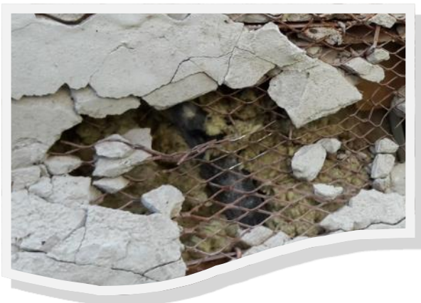
Fig 1. Close up of render removal at ground floor level showing reinforcement mesh through to degraded mineral wool insulation
