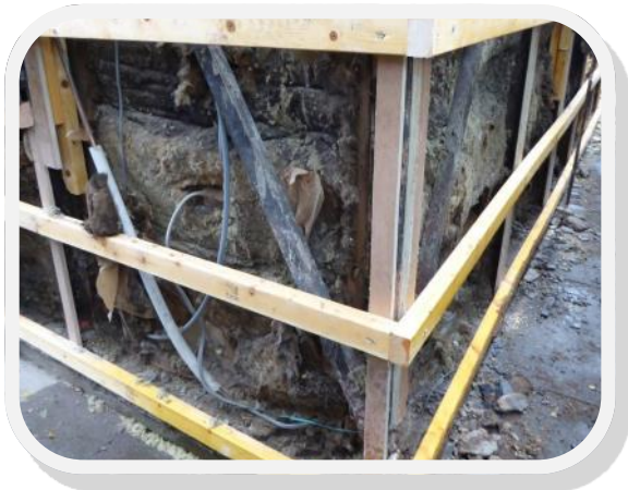
Fig 5. Timber structure applied at ground floor level to create a fixing for the ply boarding.
