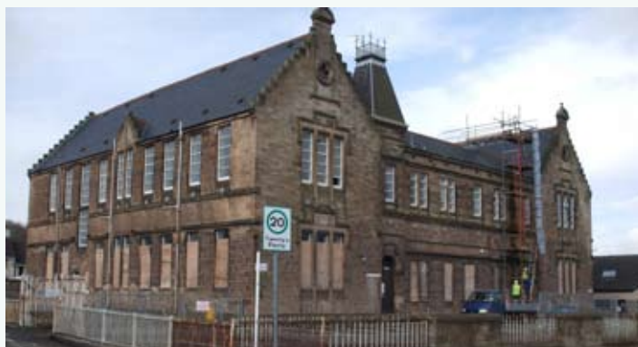
New Stevenston Primary no longer used as a School to be converted into Flats with 4 semi-detached houses to be built in the playground.
